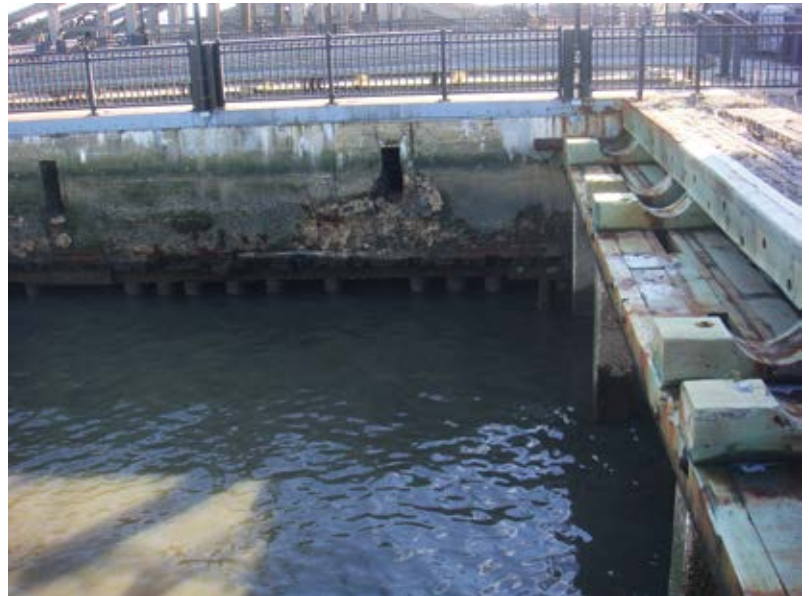
Fig. 3: Spalls along the outside wall of the Ferry House Platform #2
