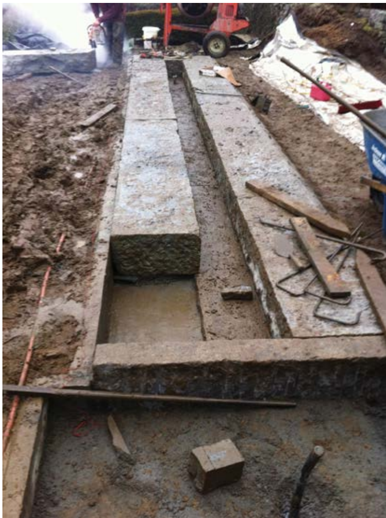
Fig. 3: Shotcrete trough with reclaimed granite installed. Notice the shotcrete step support for granite stones
