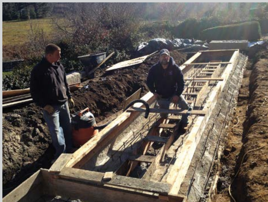
Fig. 2: Image depicts raising the installed shotcrete with a second day of shooting (no expansion joints, no bonding agents, no cold joints)
