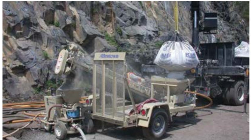
Fig. 3: Use pre-dampening equipment to reduce the amount of airborne dust at the machine and at the nozzle
