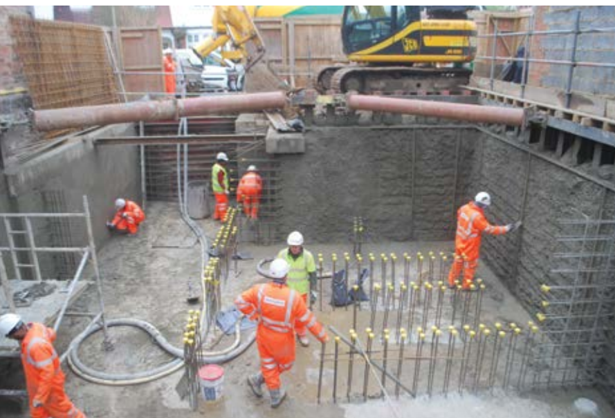
After a unique piling system was developed and implemented for this project, shotcrete containing KIM crystalline waterproofing admixture was applied to the slab and walls of the basement (Photo courtesy of Abbey Pynford—Basement Engineering Specialists)
