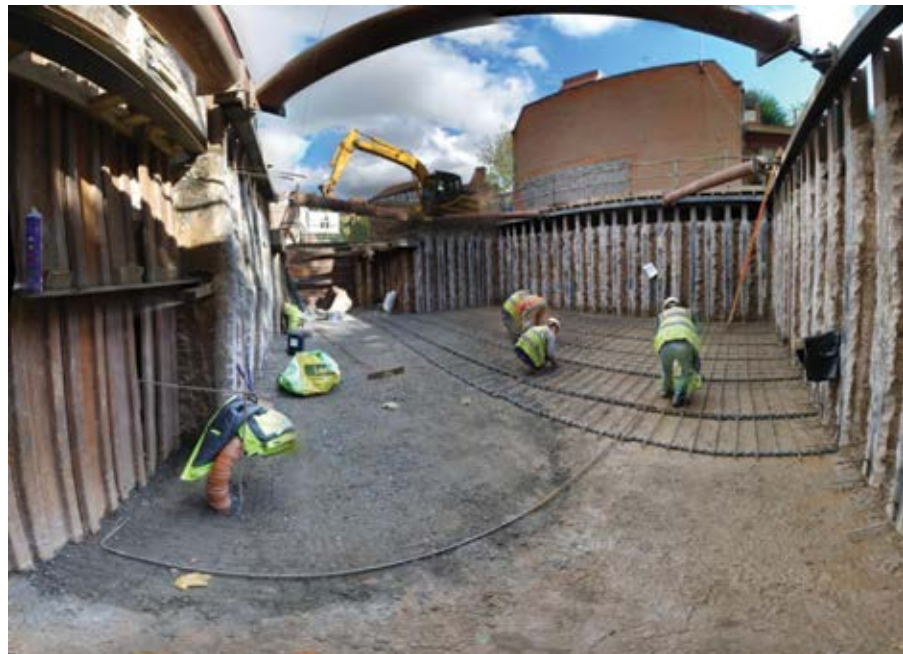
Using shotcrete and KIM together allowed the basement to be constructed right to the property line without affecting the neighboring homes (Photo courtesy of Abbey Pynford—Basement Engineering Specialists)
