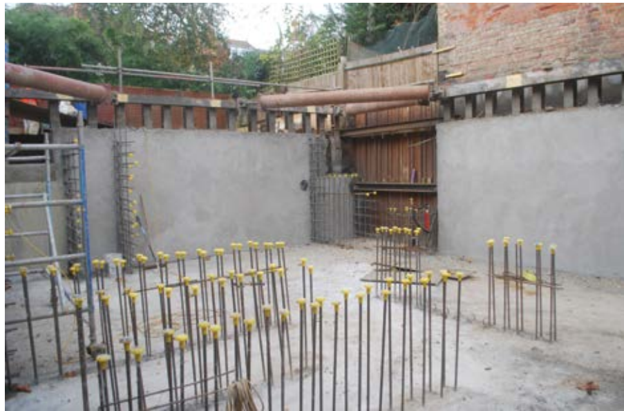
The integral crystalline waterproofing method also improved the shotcrete mixture's workability and gave the finished product a smoother architectural appearance (Photo courtesy of Abbey Pynford—Basement Engineering Specialists)
