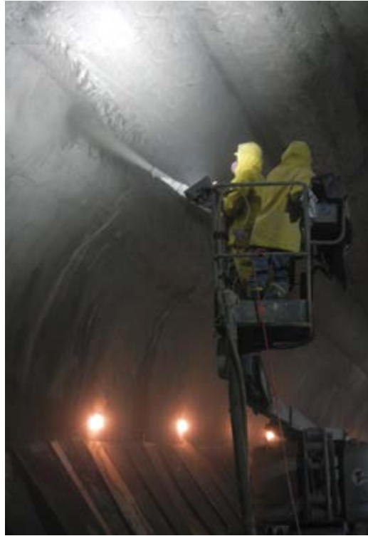
Fig. 3: Over 1200 tons (1010 tonnes) of King MS-D3 Accelerated Macro-Synthetic Fiber Reinforced Shotcrete were applied throughout the 550 ft (170 m) tunnel using an Aliva AL 252 dry-mix shotcrete machine
