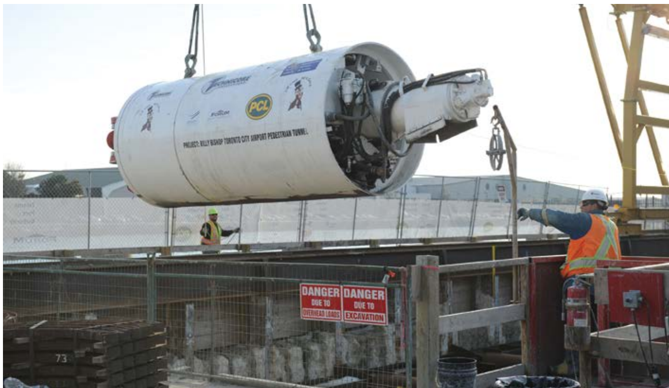
Fig. 2: Two purpose-built, Canadian-made tunnel-boring machines, dubbed “Chip” and “Dale,” were launched to bore the seven interlocking “tunnel drifts,” forming the unique arched crown design of the main tunnel
