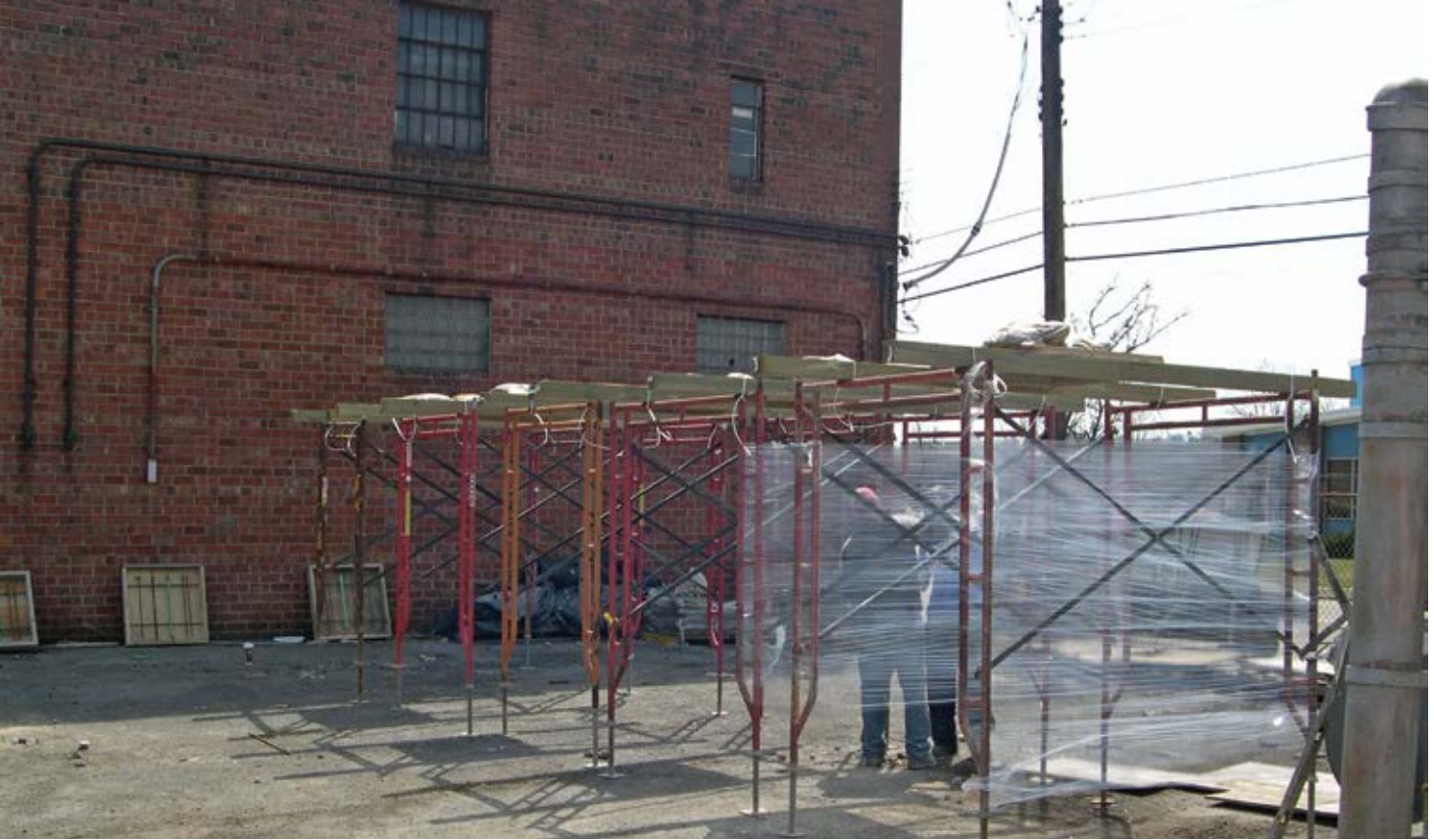
Fig. 1: Overhead panels prepared prior to the day of shooting, braced and set in an orderly fashion
