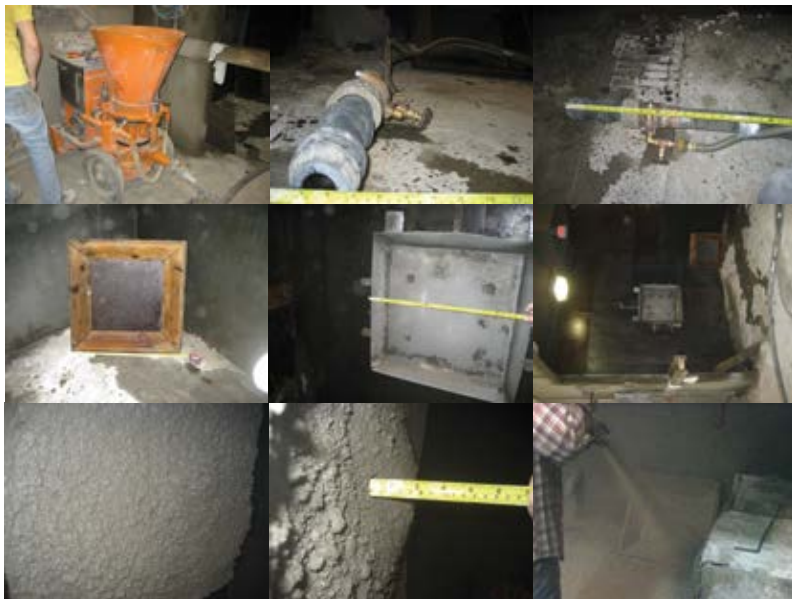
Fig. 2: Aliva 246, material and operator on scale (top left), double bubble nozzle (top middle), short hydromix nozzle assembly (top right), shotcrete panels (middle left), rebound panel (middle middle) and shooting area overview (middle right), fresh control mixture on rebound panel (bottom left), measuring buildup (bottom middle), shooting control mixture panel (bottom right)
