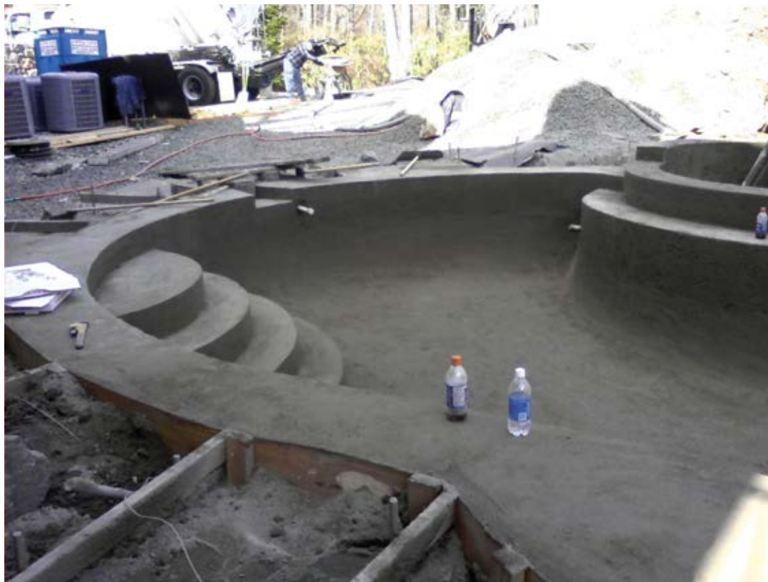
Fig. 7: Proper Steeltex forming allows the shotcrete crew to focus on their placement and finish details
