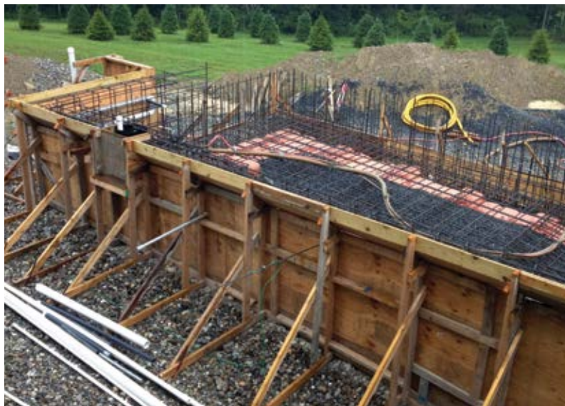
Fig. 3: A significant set of wood forms, well-reinforced, for a negative-edge pool being built above grade
