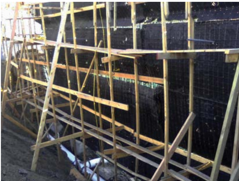
Fig. 5: A 13 ft (4 m) tall pool wall with Steeltex® hung haphazardly, with a terrible lack of support by undersized and insufficient wood forms
