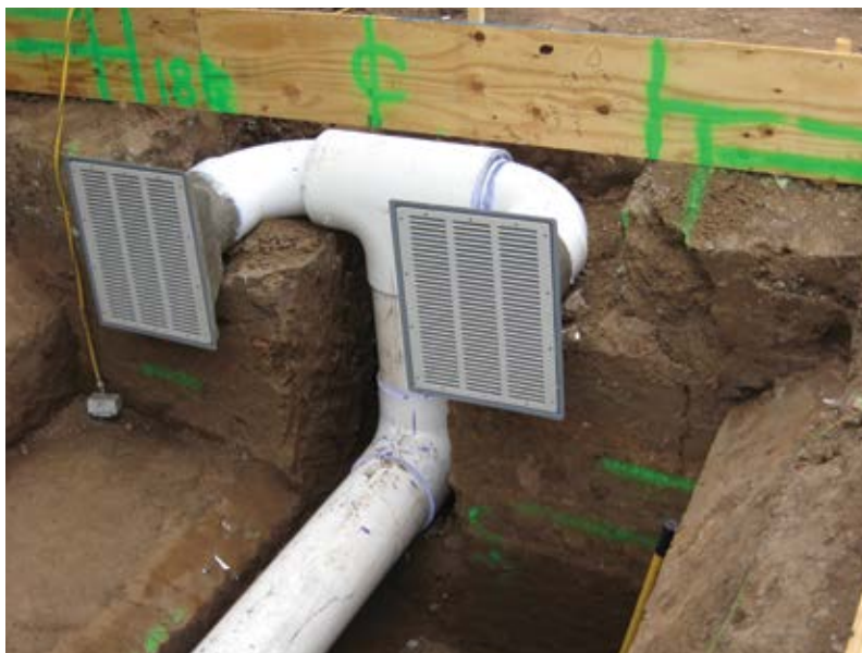
Fig. 1: The subgrade has been carved to the profile required, including trenching of plumbing lines beneath the future pool shell
