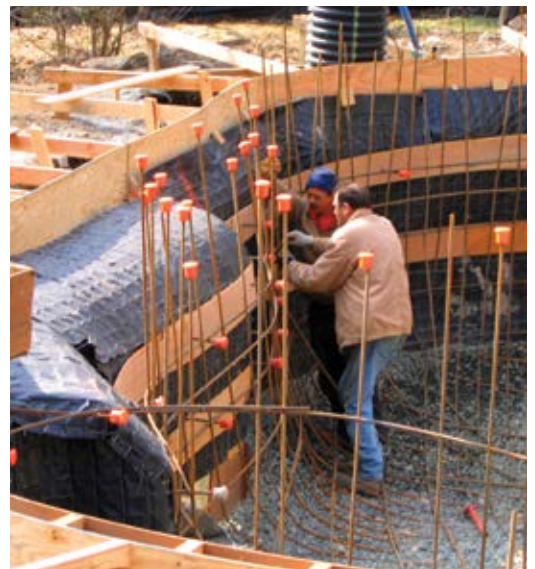
Fig. 6: Steeltex forms properly set with overlaps, wood staking behind, and plywood ribs attached to the front
