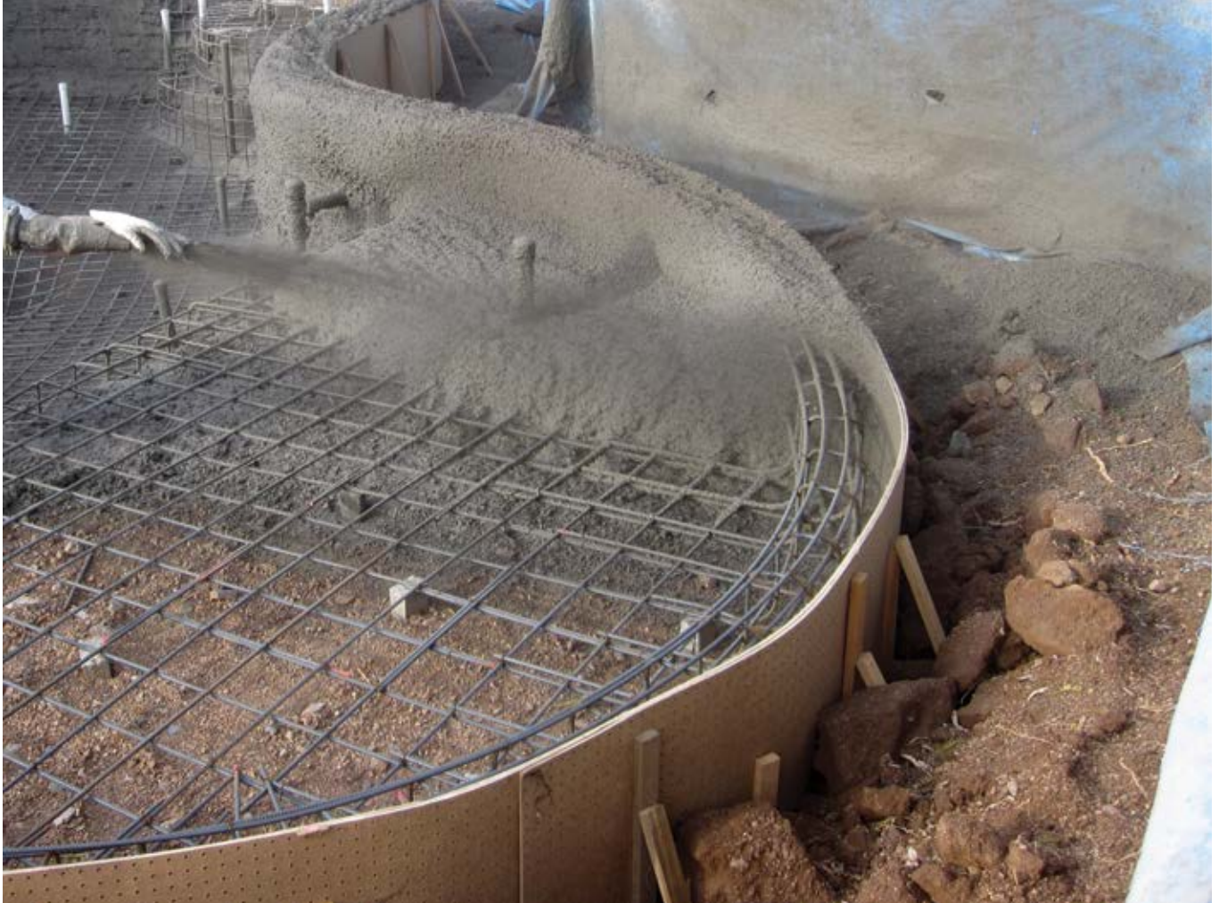
Fig. 4: Short pegboard forms poorly supported with undersized staking allows for movement at the top of forms during shotcreting
