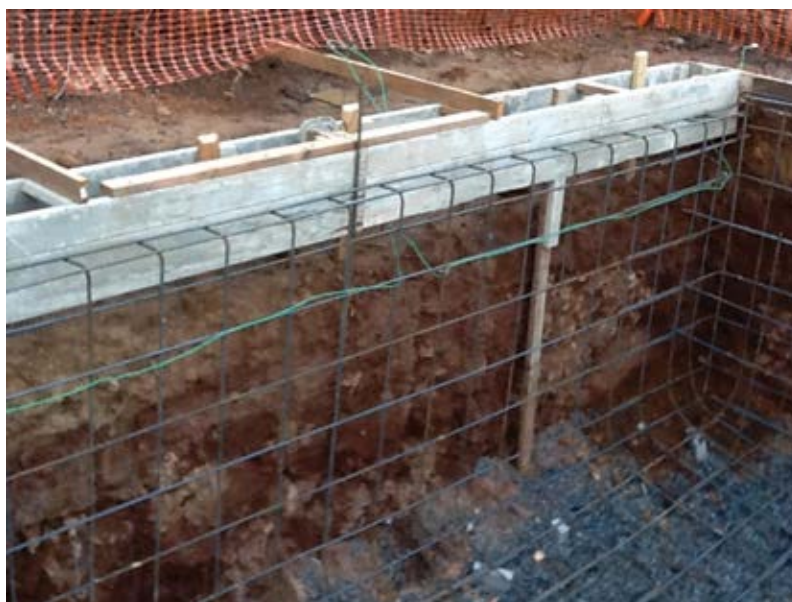
Fig. 2: The rocky soil has been trimmed to accept the shotcreted pool shell
