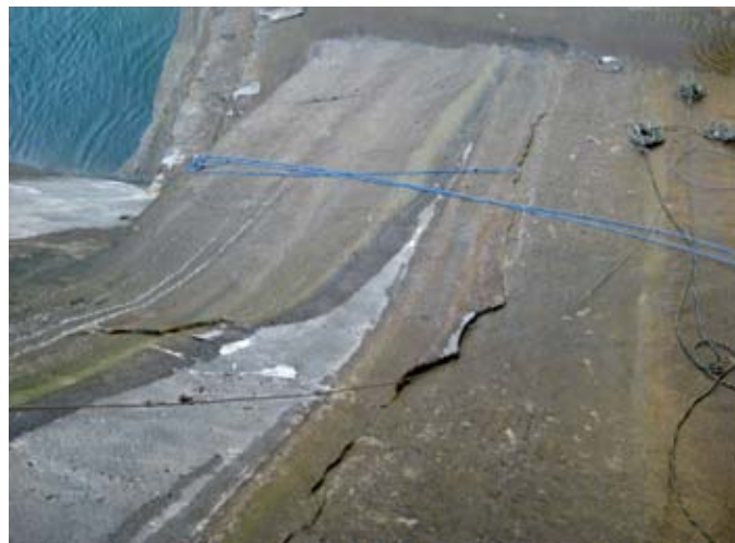
Fig. 7: Feathered edge construction joint delamination
