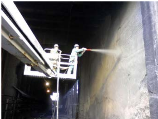
Shotcrete is easily conveyed directly to where it is needed, as shown in this shotcrete repair of the upper wall area of this Coke Plant Quench Tower
