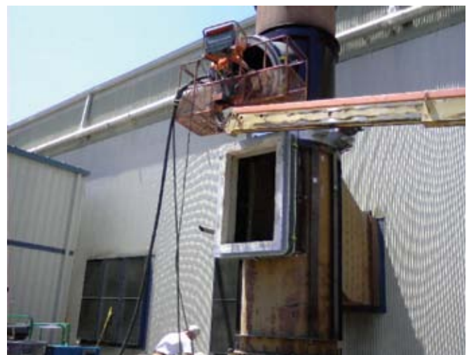
The shotcrete hose running up into the smokestack conveys the refractory material directly to the areas where it is sprayed in place. This can easily be accomplished without the double handling of materials that would have been necessary with the installation of refractory brick
