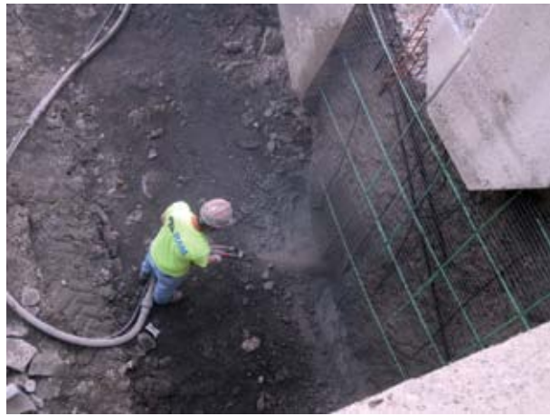
The structure required a significant number of repairs, some of which required up to 14 in. (356 mm) of concrete replacement
