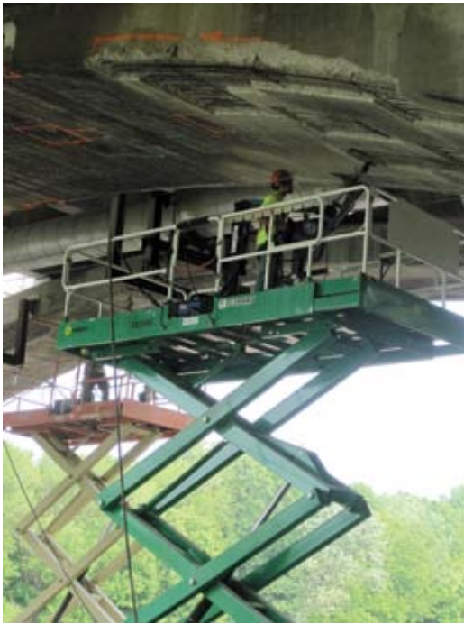
Repair access on the underside of the bridge spans using scissor lifts
