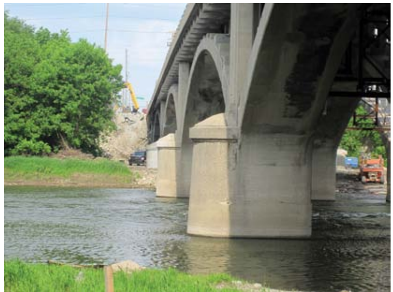
RAM's scope of work called for rehabilitation of abutment walls, wing walls, arch spans, and piers
