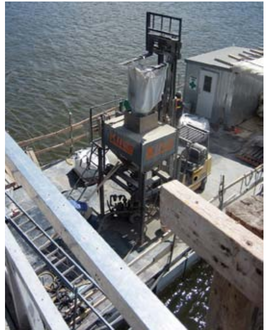
Silos are loaded with shotcrete material by a forklift on the barge for continuous and efficient material flow. The shotcrete material was lifted to the barge by crane
