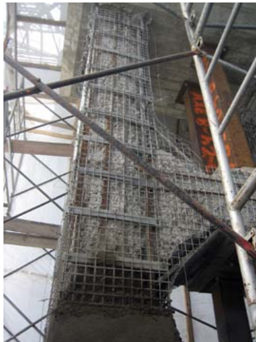
The column was chipped to 1 in. (50 mm) behind the corroded rectangular steel reinforcements, cleaned, and covered in a welded-wire steel mesh
