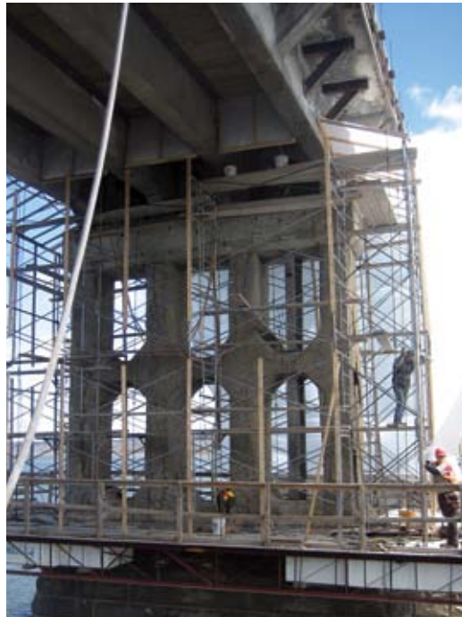
Scaffolding before chipping has begun. The limestone masonry and map-cracking on the existing concrete is also visible
