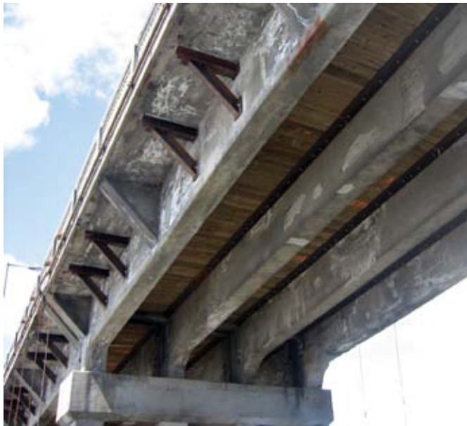
The concrete beams and timber deck are clearly visible, showing how various materials can work together. Some salt stains, corrosion, and freezing-and-thawing damages show how materials age
