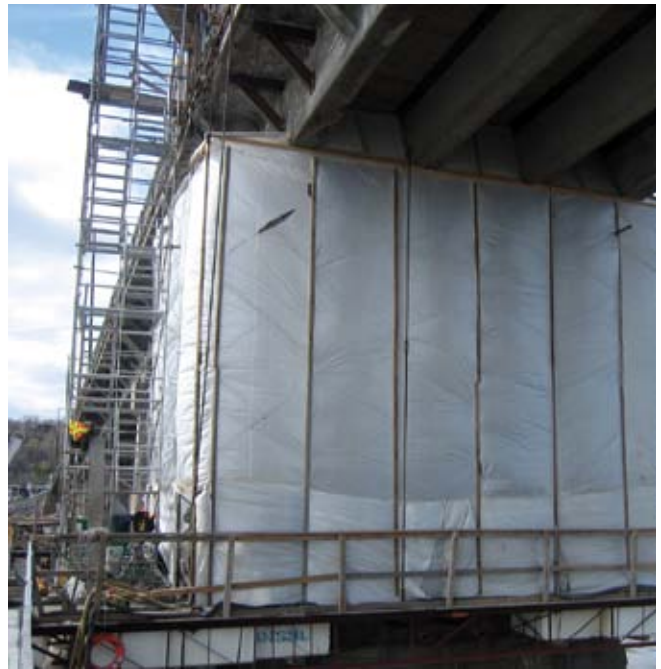
The shotcrete workspace was protected from wind, while also preventing dust and debris from falling into the river
