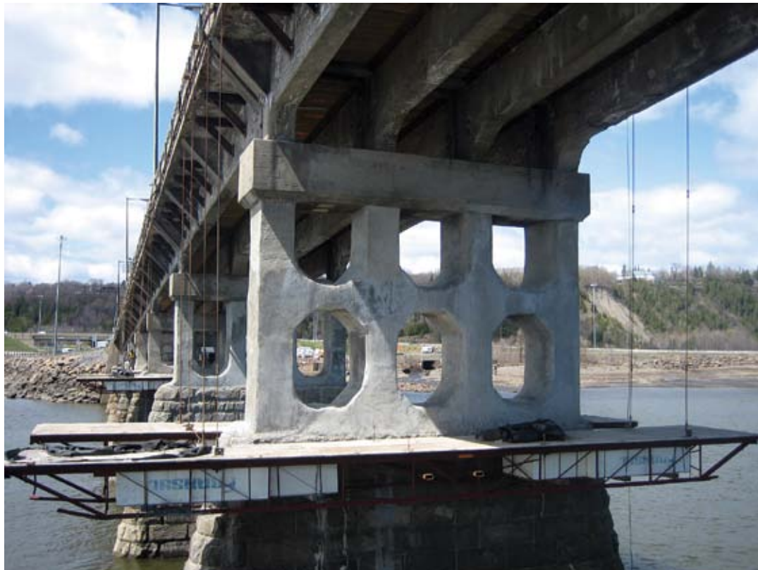
A finished repair is visible, with a support platform in place for final touches and inspection
