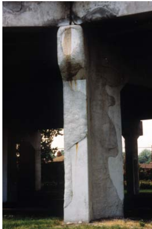
Until 1989, the MTO specification allowed for site mixing, which often led to inconsistencies in mixture proportions. Inconsistent cement contents would often lead to high shrinkage values, which contributed to cracking and debonding
