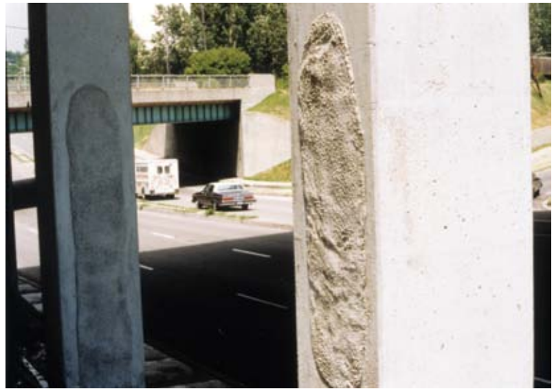
The specification for latex-modified shotcrete required that hand finishing be minimized, leaving the repair with a gun finish
