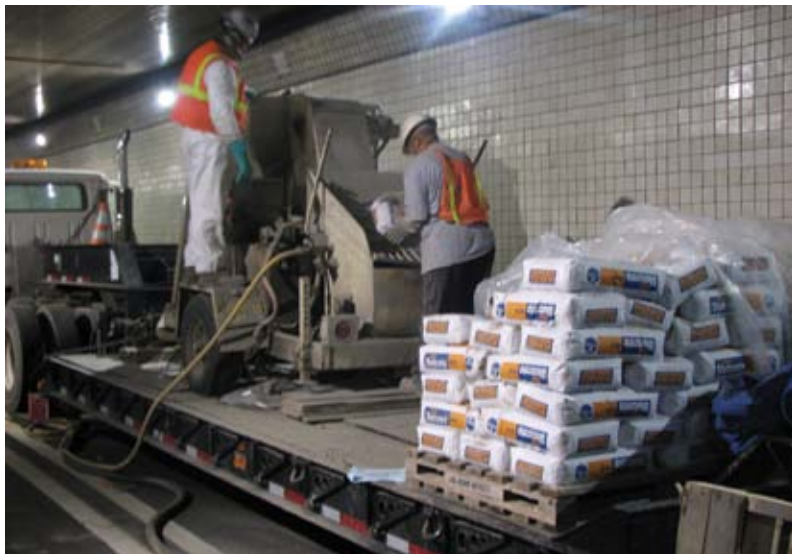
The current MTO shotcrete specification allows for only prepackaged materials with performance test data verifying that the material meets the requirements of the specification
