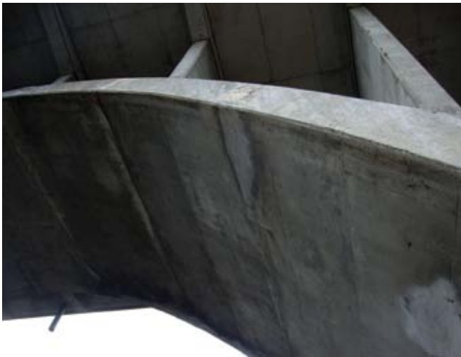
After 21 years, there was no evidence of debonding or failure in any of the shotcrete patches of the Magnetawan River Bridge structure
