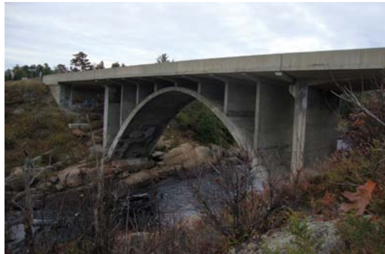
The success of the Magnetawan River Bridge project led to the development of the current MTO shotcrete specification
