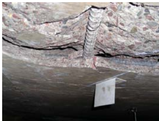
Crack in roof
