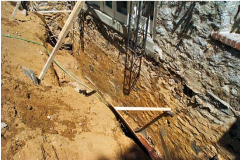
Foundation exposed down to footing drains
