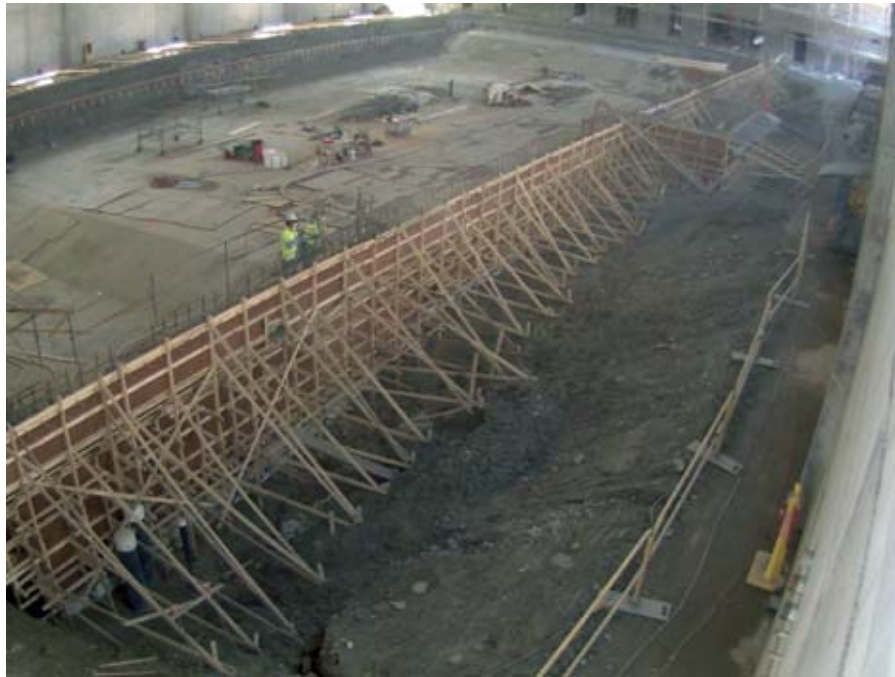
Fig. 4: Shotcrete in progress. This pool required significant formwork, as 85% of the pool was 9 ft (3 m) deep or deeper
