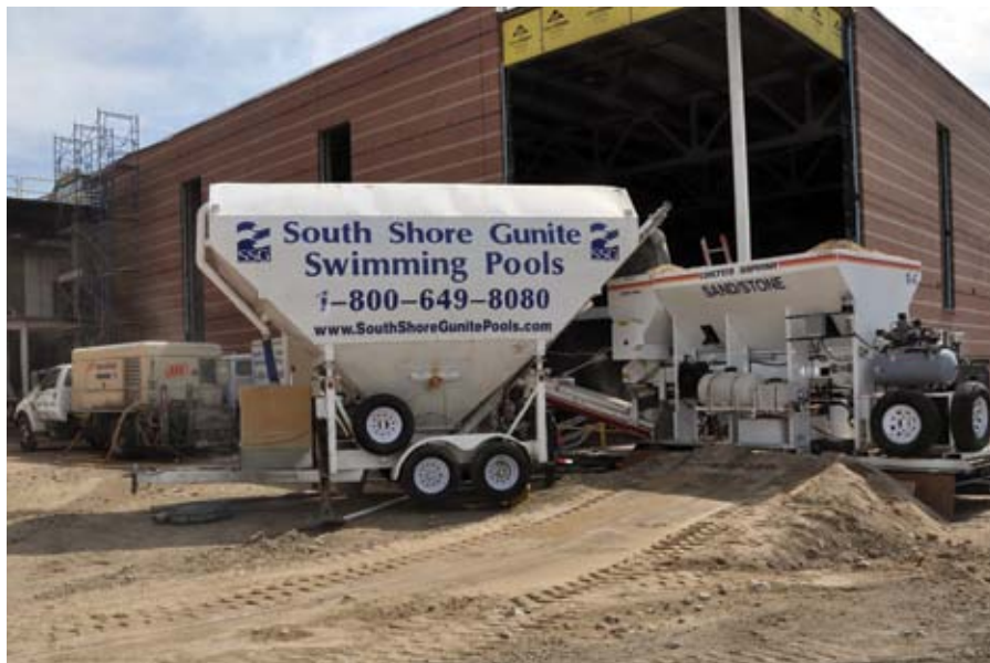
Fig. 5: The shotcrete mixture was made on site using a portable cement silo and a volumetric batch plant. This saved on material costs, allowed us to control our mixture and material delivery, and eliminated concerns regarding possible breakdowns with a concrete truck. Also shown is the truck-mounted 825 CFM air compressor
