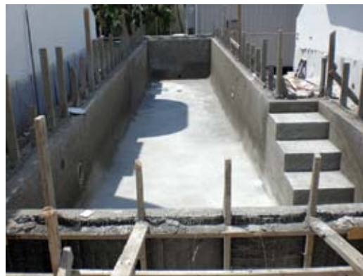
Fig. 7: Dry-mix process with use of Steel Tex in the foreground. Residential lap pool, West Palm Beach, FL
