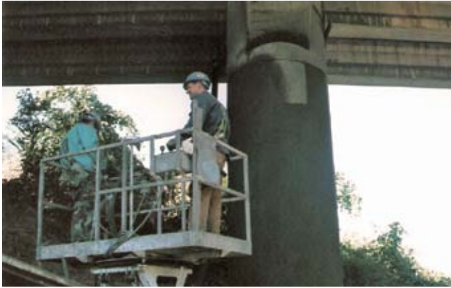
Shotcrete can easily conform to rounded or irregular shapes and varying depths, as illustrated by this freshly gunned circular-shaped bridge pier
