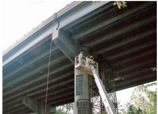
The deteriorated concrete on this bridge pier has been removed, the reinforcing bar exposed, and the surface prepared prior to the shotcrete placement. The use of shotcrete eliminates the need for forming and labor costs involved
