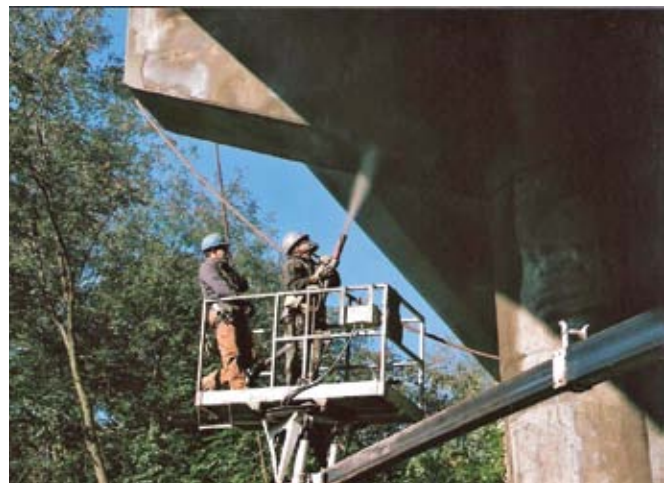
Shotcrete can be efficiently gunned overhead in concrete repair applications, where forming and material placement can be difficult and expensive, as evidenced by this dry-process shotcrete repair
