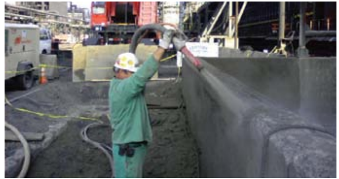
In this dry-process shotcrete repair of an industrial sump, the repair mortar is gunned in place without the need to make or install forms
