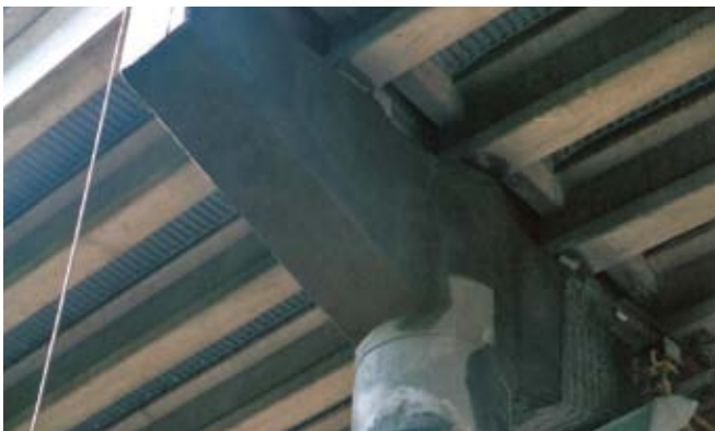
On this pier hammer head, the shotcrete is easily gunned in place without the need for forming
