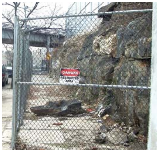
Fig. 1: Initial condition—fallen rock
