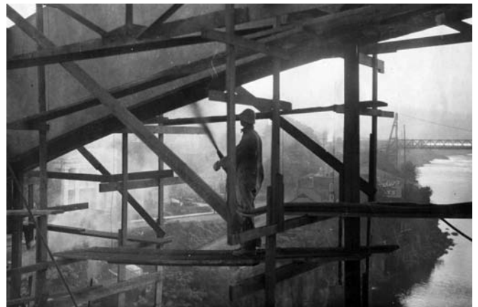
Oregon City Bridge during construction Photo courtesy of the Oregon Department of Transportation
