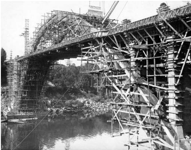
Oregon City Bridge during construction Photo courtesy of the Oregon Department of Transportation
