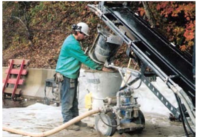
Fig. 4: Dry-process equipment and operator during the shotcrete installation of an underground culvert
