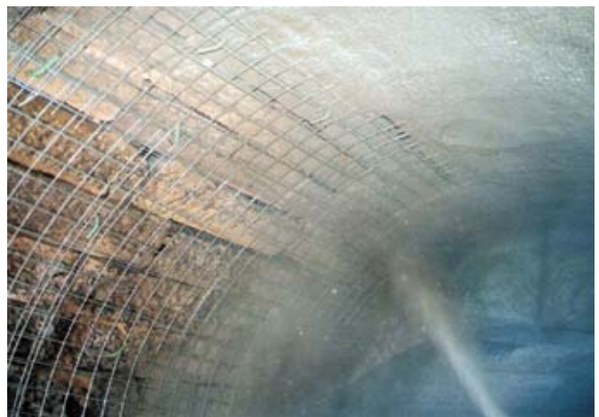
Fig. 5: Dry-process shotcrete being gunned overhead in an underground culvert. The roadway was opened the following day
