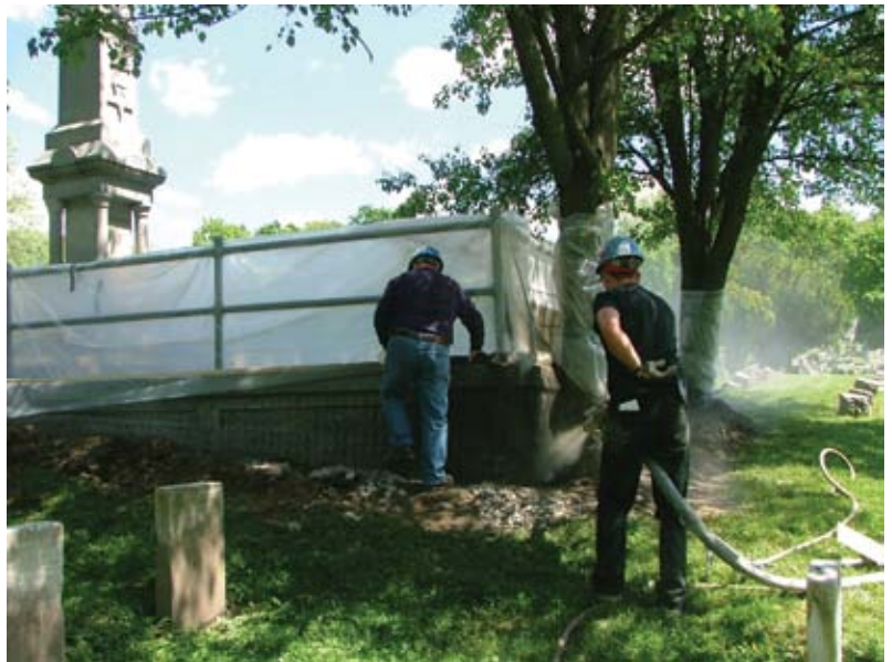
Fig. 4: After the deteriorated concrete was chipped out, the surface was prepared and meshed and the shotcrete was gunned in place
