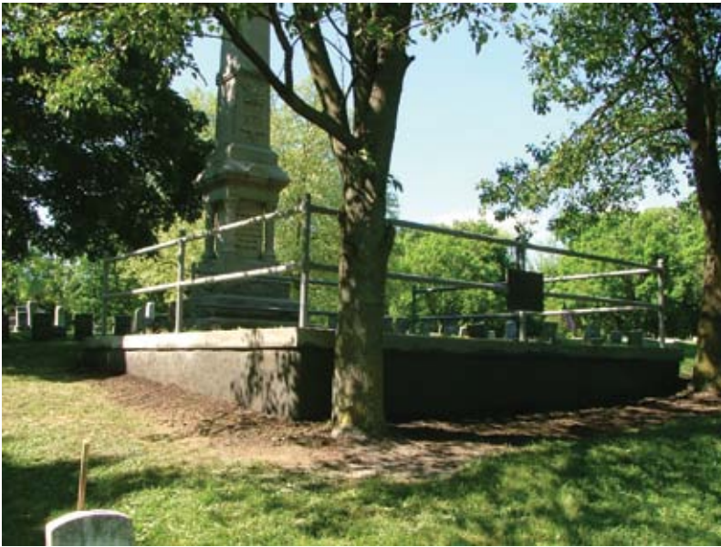
Fig. 6: A side view of the Civil War monument after the completion of the shotcrete work
