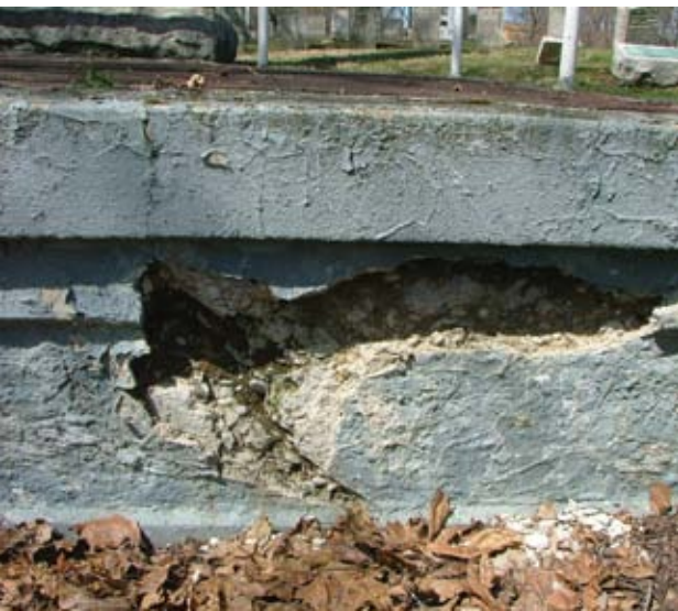
Fig. 2: The foundation wall of the Civil War monument's review stand at the Chartiers Cemetery was badly deteriorated
