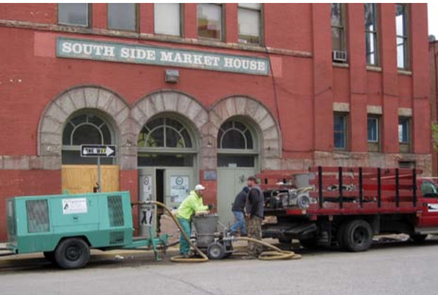
Fig. 1: The shotcrete crew prepares to start in front of the South Side Market House in Pittsburgh, PA. The structure, which was built in 1893, is listed on the National Register of Historic Places
