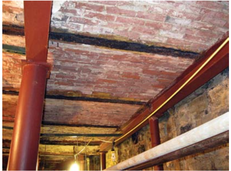
Fig. 3: These brick arches are in one of the open sections of the supporting floor system
