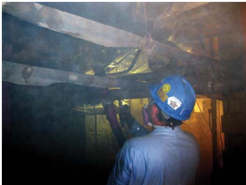
Fig. 6: The nozzleman is placing shotcrete overhead in an especially congested area of the basement behind the elevator shaft
