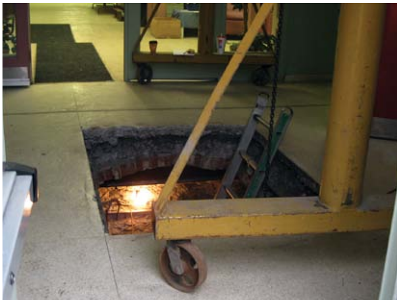
Fig. 2: In this access hole, which was cut to gain access into the building's basement, a side view of a supporting brick arch is visible
