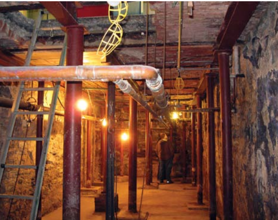
Fig. 5: Working around the structural supports, piping, conduit, and other obstructions added to the difficulty of the overhead shotcrete placement
