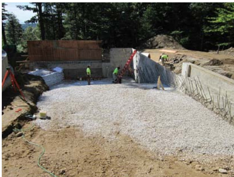
Fig. 1: Stone underlayment along with the reinforcing bars penetrating out of the first phase of construction so the second-phase pool section could be tied in correctly
