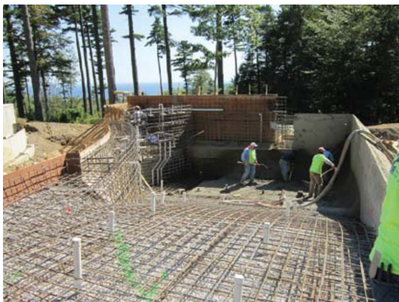
Fig. 2: Elaborate reinforcing required by the pool design as we start the second phase of shotcrete
