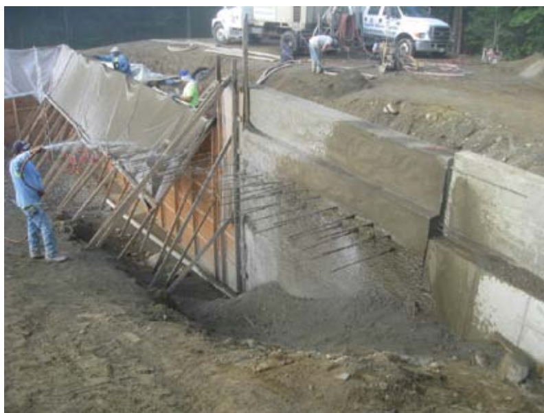
Fig. 3: Deep excavation required for forming and, subsequently, filling with free-draining stone to prevent frost heave. Also seen is the dowel reinforcing bar that was tied into the pool floor in the second phase
