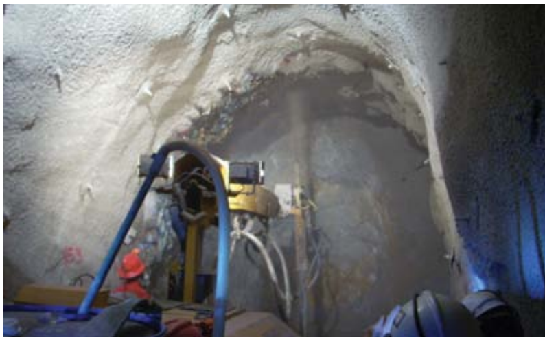
Fig. 2: Sprayer starts at bottom of wall on right and sprays up, over, and down the opposing wall—overspray is deposited on the left side wall
