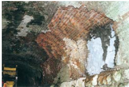
Fig. 4: Large repair area prior to shotcrete
