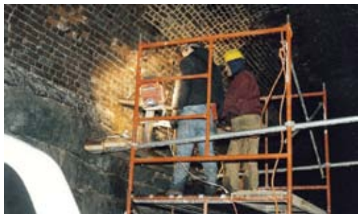
Fig. 3: Trailer-mounted core-drilling setup for drilling holes for drainage pipes. Also note the freshly repointed brick mortar joints
