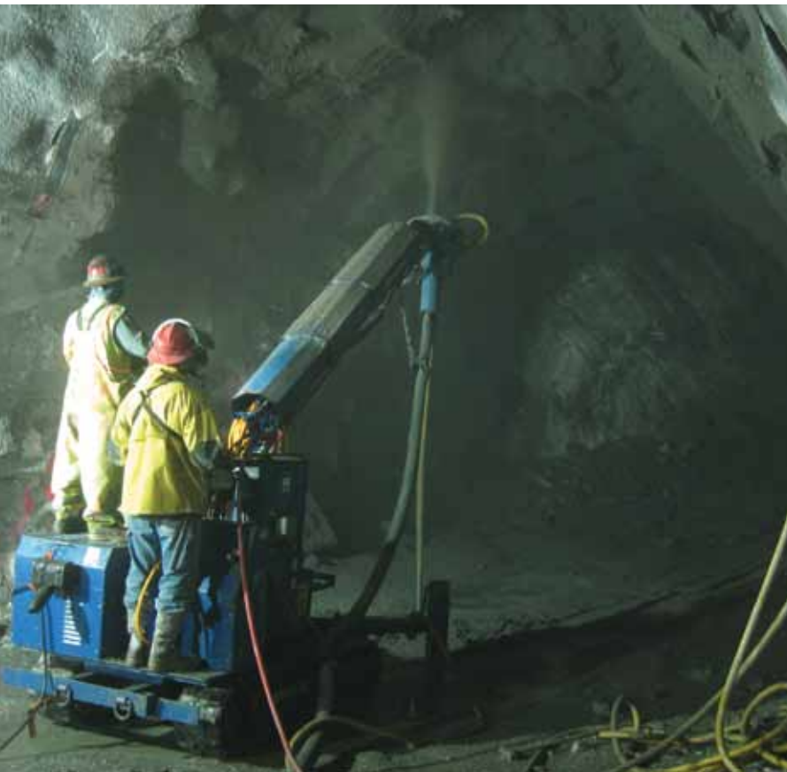
When shotcreting underground, the nozzle operator must address joints in the rock and assure proper coverage to provide support to the ground
