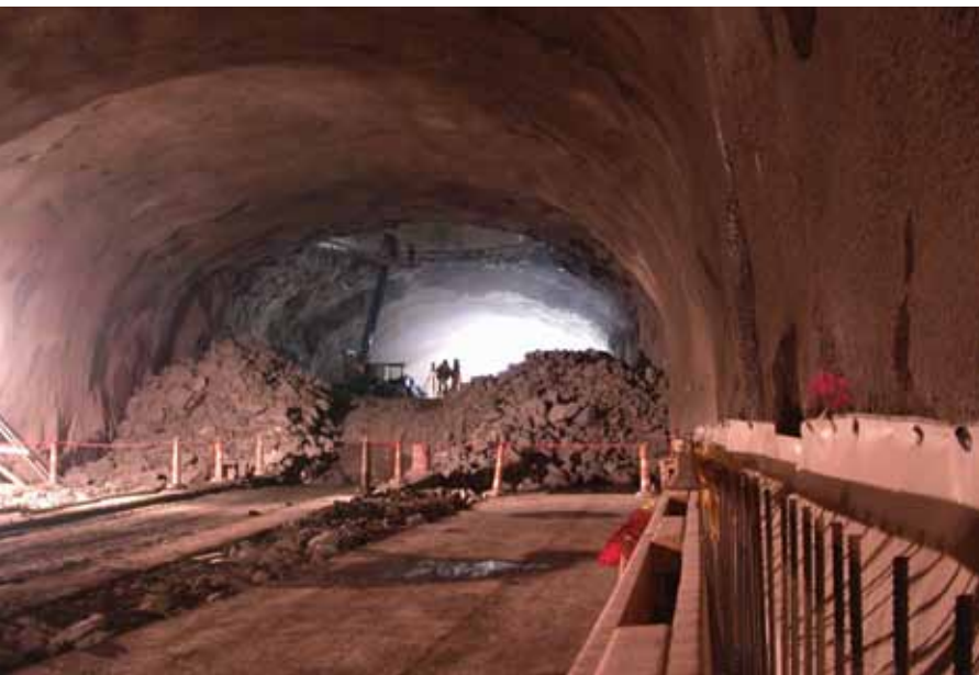
Today, nearly all tunnels under construction in North America will use shotcrete as part of their support system
