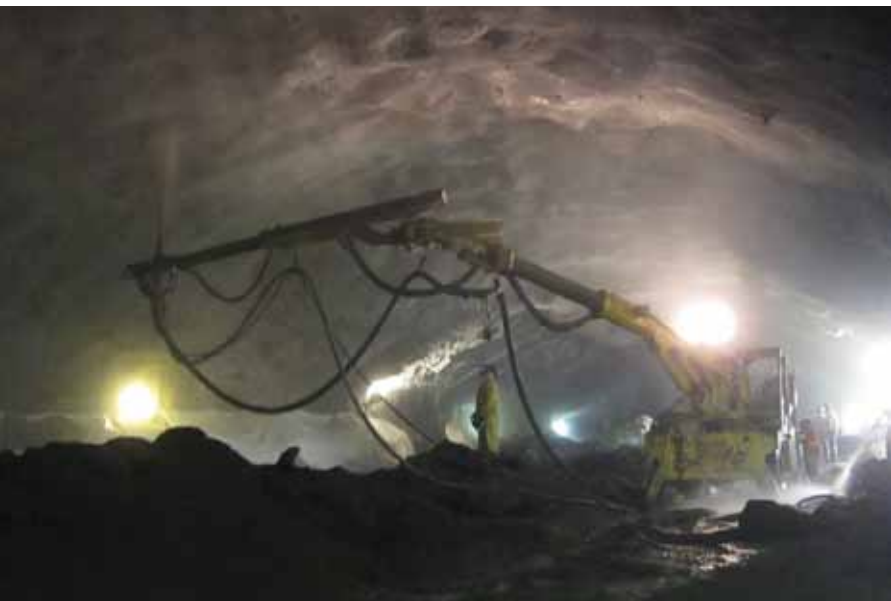
Modern transit projects require large caverns for stations. Shotcrete and modern shotcreting equipment make this possible
