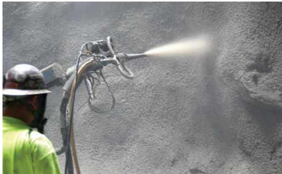
To ensure proper adhesion on vertical and overhead surfaces, set accelerators are introduced into the nozzle to alter the setting characteristics of the shotcrete
