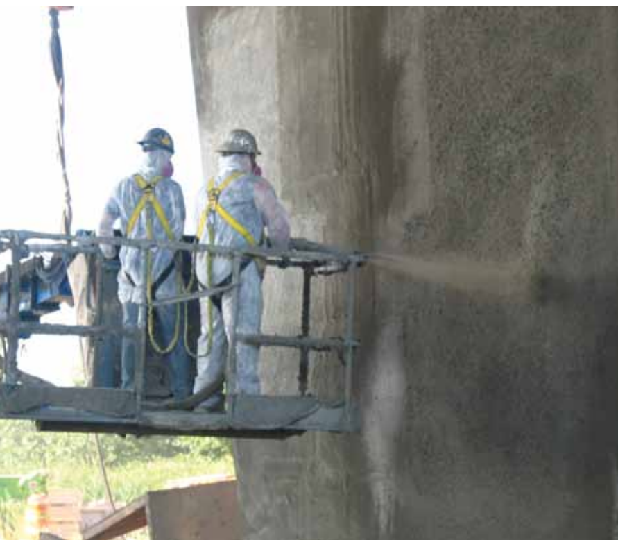
Since 1989, the Ministry of Transportation of Québec has included the use of 3/8 in. (10 mm) aggregates in its dry-mix shotcrete specifications
