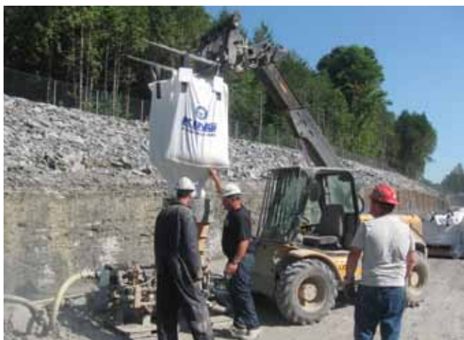
Fig. 4: The flexibility offered by preblended, bulk-bag materials also allowed the shotcrete crew to carry an inventory of shotcrete material on site
