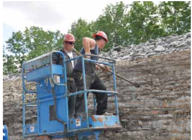
Fig. 5: Prior to the application of shotcrete, rock anchors were installed in a staggered vertical 5 ft (1.5 m) by horizontal 5 ft (1.5 m) pattern
