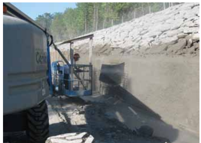
Fig. 6: An ACI-certified nozzleman was part of the shotcrete crew, as specified by the design engineers
