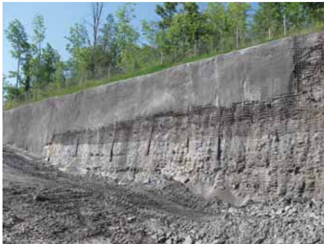
Fig. 3: Option 4 was the only feasible option for the area along the west wall of the canal where there was minimal available land between the power canal and the river
