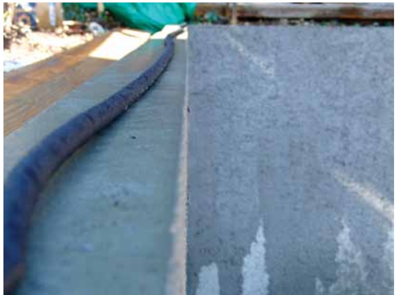
Fig. 2: A soaker hose can be useful in establishing saturated conditions prior to the application of an additional layer of shotcrete
