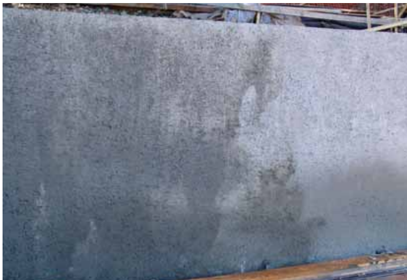
Fig. 4: Wall section at left is in SSD condition. Section area at right has lost SSD condition; additional moisture must be applied to right section prior to shotcrete application
