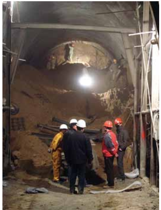
The side wall and base construction follow once the tunnel is excavated
