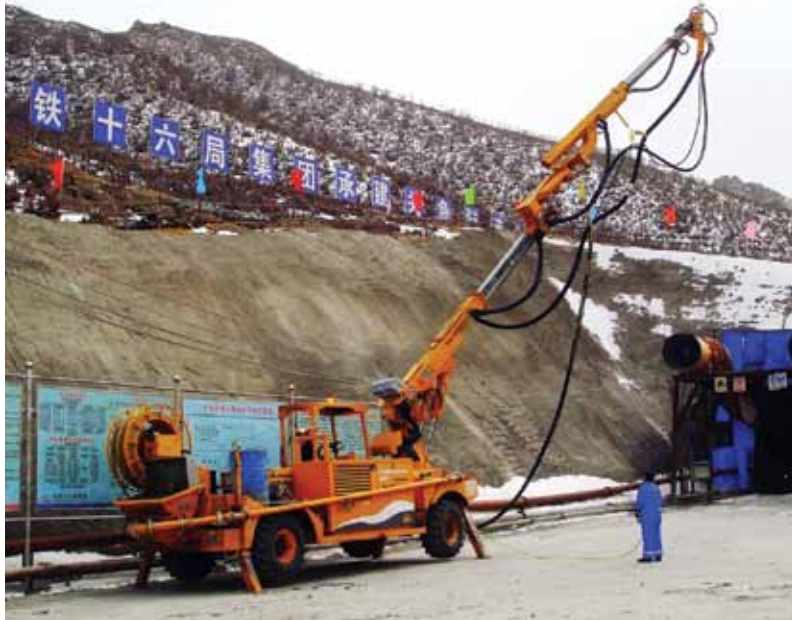
This operator familiarizes himself with the remote control of the modern concrete-spraying system
