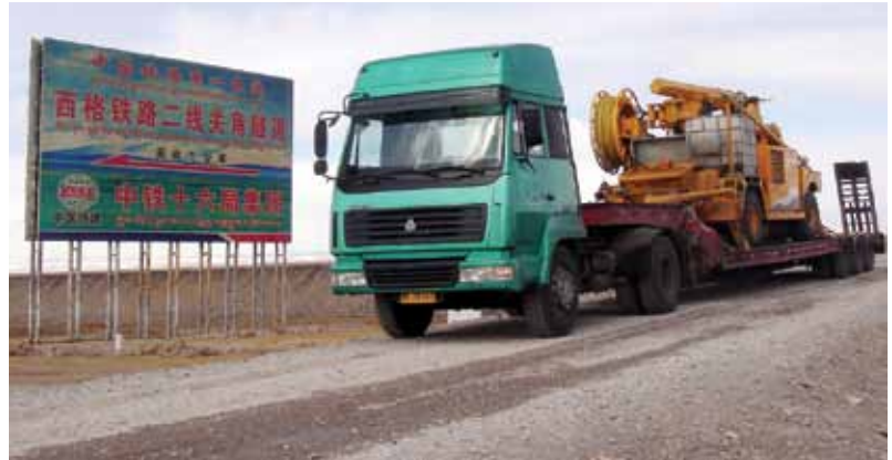
Transport of the shotcrete unit crossing a pass situated at an altitude of about 11,843 ft (3500 m)
