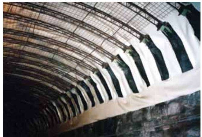
Note the horizontal wire at the bottom of this picture—this is the ground wire for one set of tracks. A similar wire was installed for the other set of tracks
