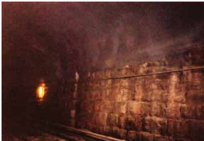
The third rail is located about a foot up from the bottom in this picture
