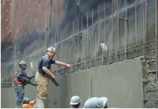
In many cases, when there is a structure or substrate to gun against, shotcrete can be gunned in place without the use of forms, eliminating forming costs altogether
