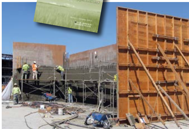
Shotcrete sprayed in place against one-sided forms saves 50% of the forming required in cast-in-place installations
