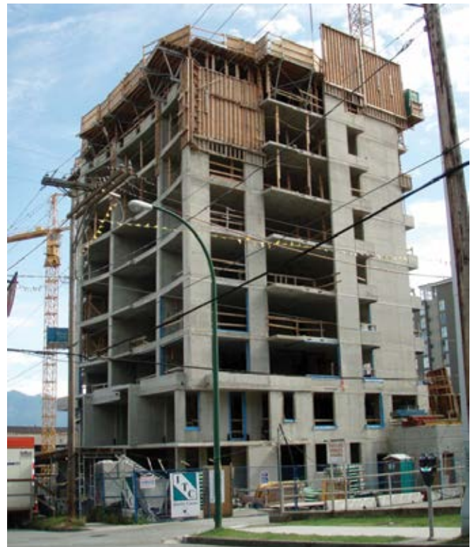
Panels are set in place on this high-rise to create one-sided backstop forms to gun shotcrete against
