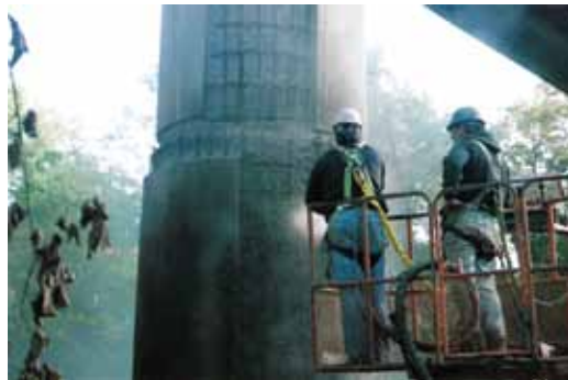
With good surface preparation and gunning practices, shotcrete provides an excellent bond to the existing substrate
