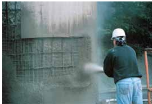
The dry process of shotcrete being gunned on a pier can provide a better bond without using bonding compounds. The nozzleman is filling in the corners first and working toward the middle of the repair area so he doesn't trap rebound in the corners
