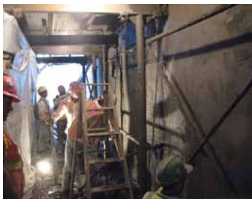
Wet-mix shotcrete was the only acceptable method the engineer would entertain to minimize and control the dust and rebound
