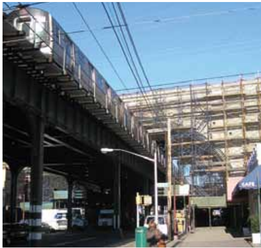
As a safety precaution, stage scaffolds and netting were erected long before the work started to protect the subway tracks and, more importantly, the pedestrians on the station platforms and sidewalks below
