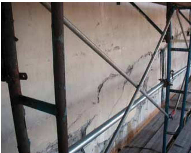
Typical minor concrete spalling
