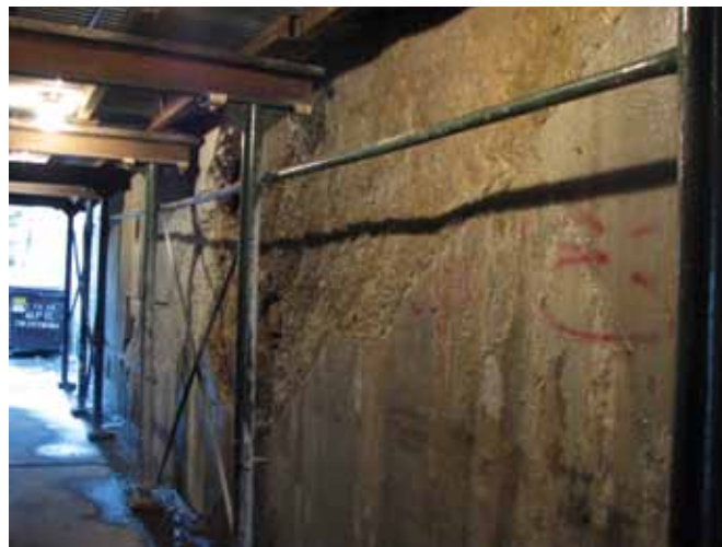
Typical severe concrete spalling with continuous groundwater infiltration
