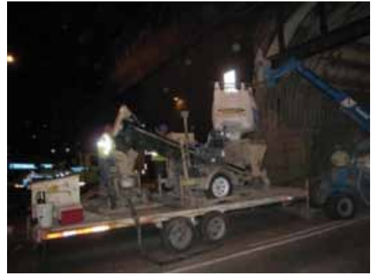
The 3000 lb (1361 kg) bulk bags were predampened as a part of the installation process
