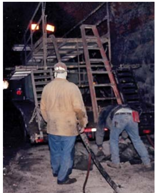
Scaffolding setup on mobile trailer with lighting for access to work. Air compressor and power unit mounted beneath scaffolding
