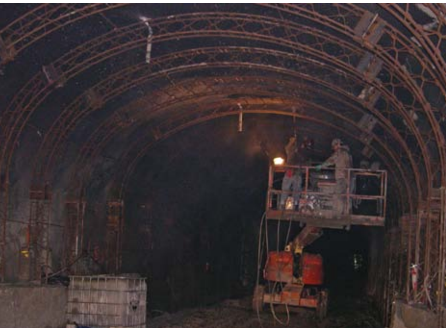
Pressure-washing being performed from the man-lift used for shotcrete, which gives a good perspective of dimensions of tunnel and access requirements
