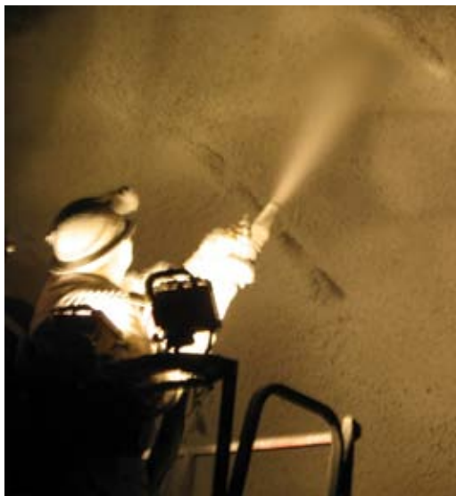
Nozzling performed from man-lift equipped with lighting, allowing for excellent visibility and immediate access to work while supporting the majority of the material delivery weight and air hoses
