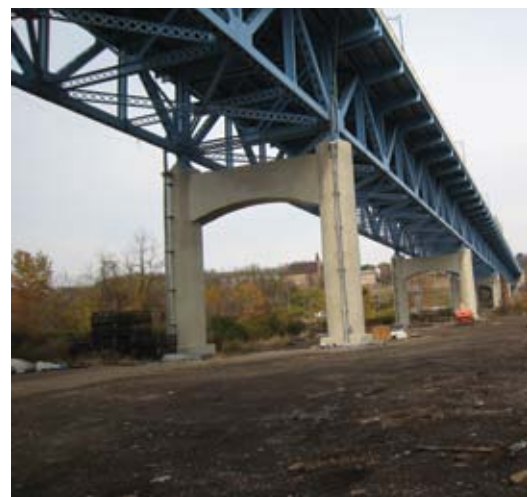
After completion of the project, the structure looks like a new bridge
