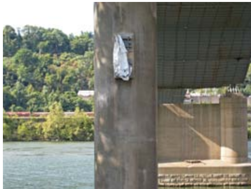
Large, round piers can be brought back to their original shape using shotcrete
