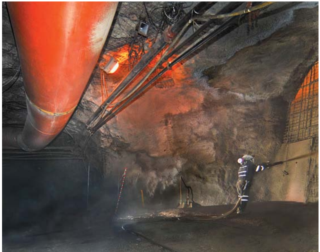
A shotcrete nozzleman should have a clear view of the rock face when applying shotcrete
