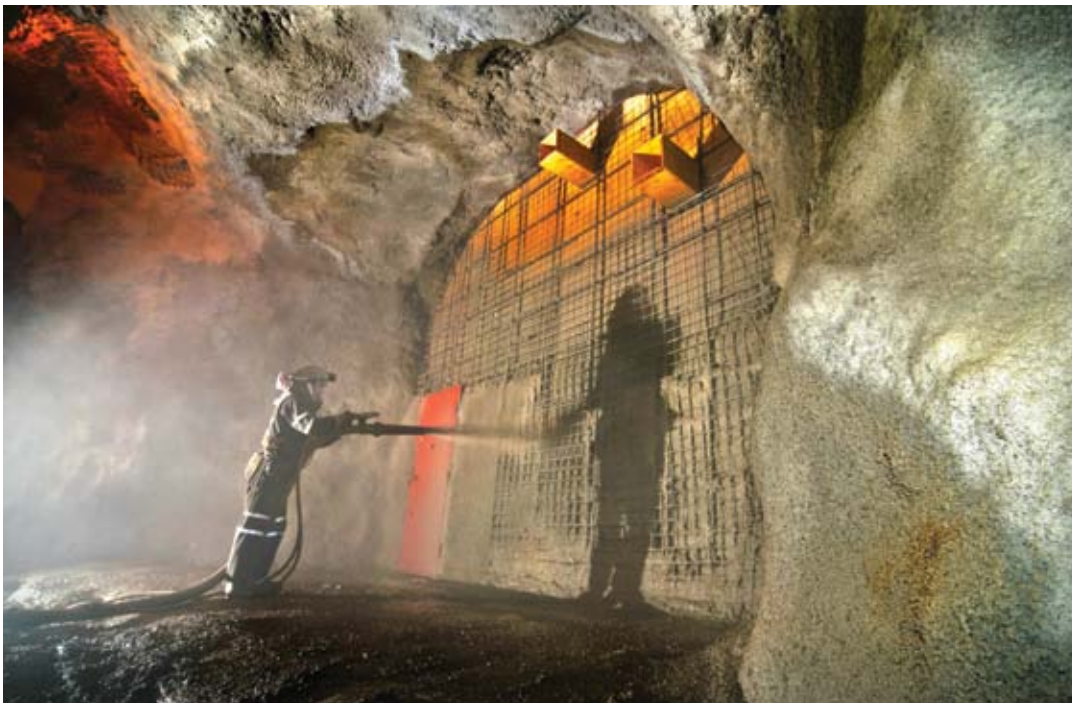
Proper lighting will reduce workplace accidents, but it is particularly important in an underground environment
