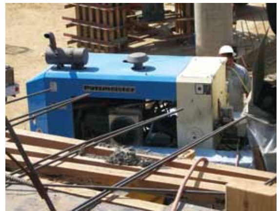
With its high-performance trailer pump and shotcreting expertise, Global Shotcrete of Ventura, CA, plans to shoot approximately 4000 total yd 3 (3058 m 3 ) of shotcrete for the walls on the large-scale project
