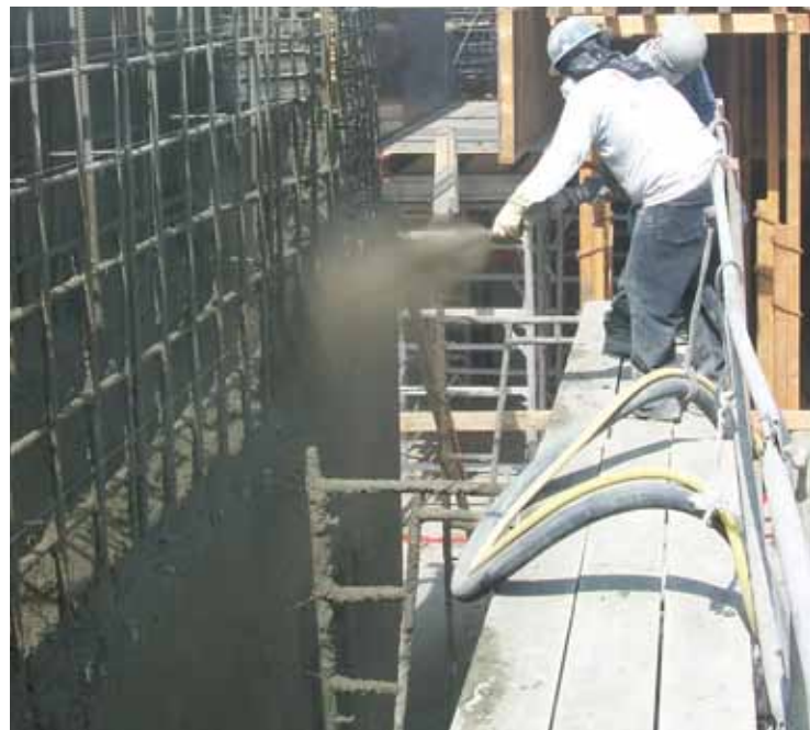
Numerous walls are being placed with shotcrete, including the exterior walls around the perimeter of the large 330,000 ft 2 (30,658 m 2 ) complex, plus all major interior walls
