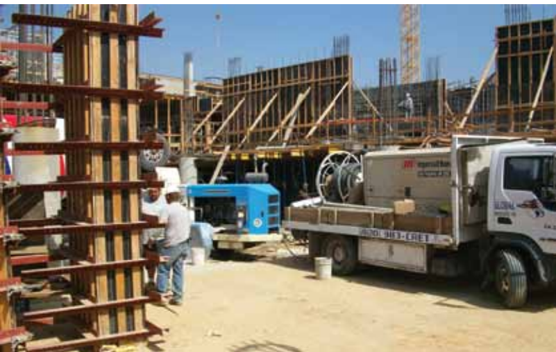
The Thom-Katt TK 50HP trailer pump is on the job site twice a week, shooting 80 to 130 yd 3 (61 to 99 m 3 ) of shotcrete during an average 8- to 10-hour day
