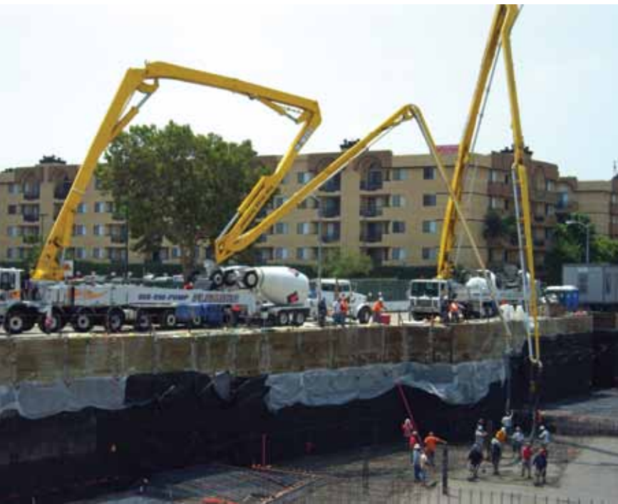
Fleming Concrete Pumping of Santa Ana, CA, is expected to pump over 65,000 total yd 3 (49,696 m 3 ) of concrete for the footings, columns, and slabs upon the project's completion
