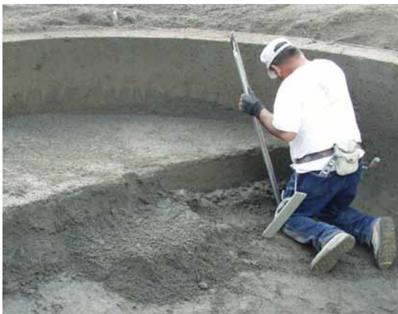
Shotcrete inspection would help eliminate many unacceptable practices such as making steps and benches with rebound
