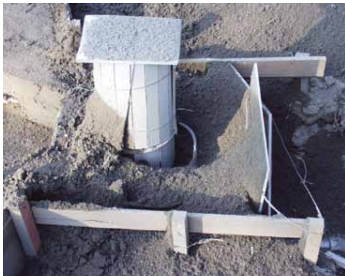
Shotcrete inspection would eliminate many unacceptable practices such as packing rebound around skimmers
