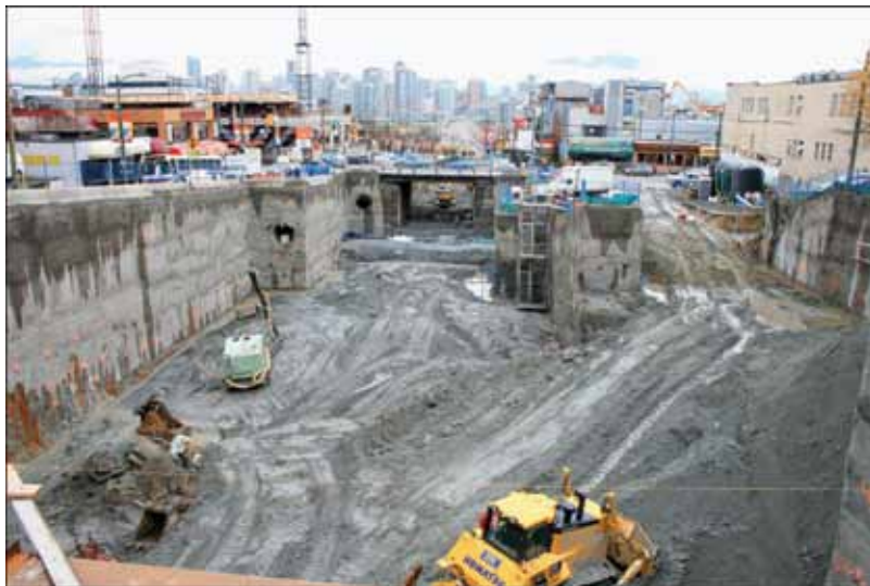
Fig. 13: Broadway Station: Note temporary bridge for vehicular traffic, which accommodated two lanes east and two lanes west along Broadway
