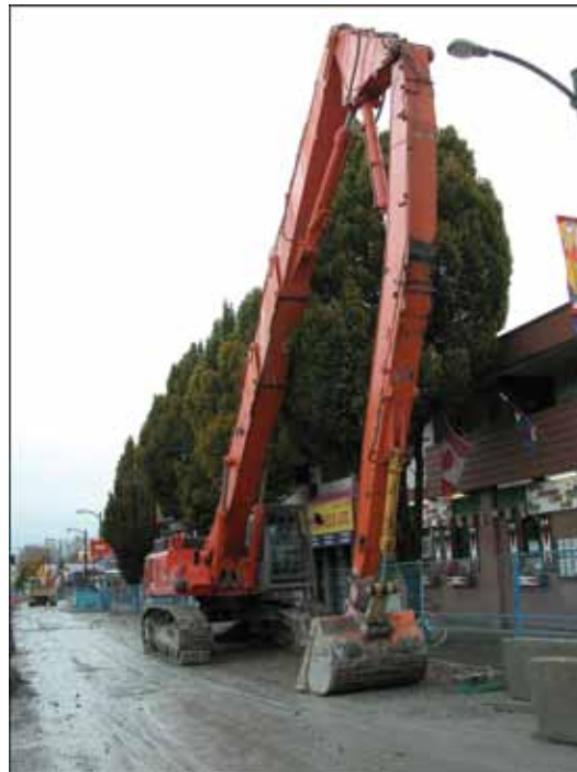
Fig. 11: Long stick backhoe, fitted with camera on underside of the boom. Monitor is in the cab
