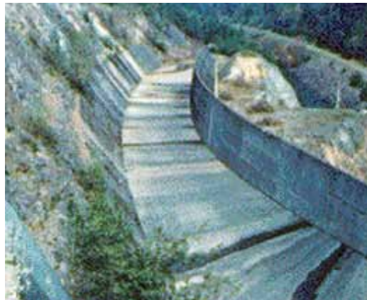
Spillway at Howard A. Hanson dam, 1990s Courtesy U.S. Army Corps of Engineers
