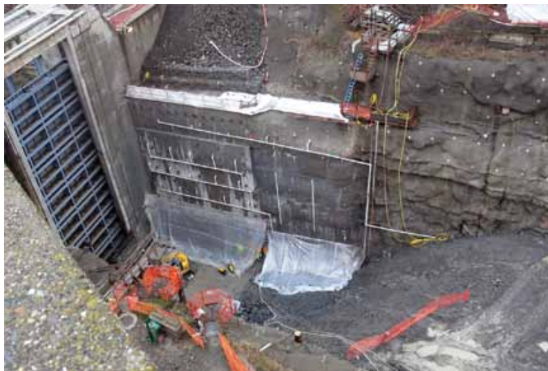
Phase I and Phase II jobs combined, as the shotcrete contractor finishes the bottom lift under the heat tent during Phase II
