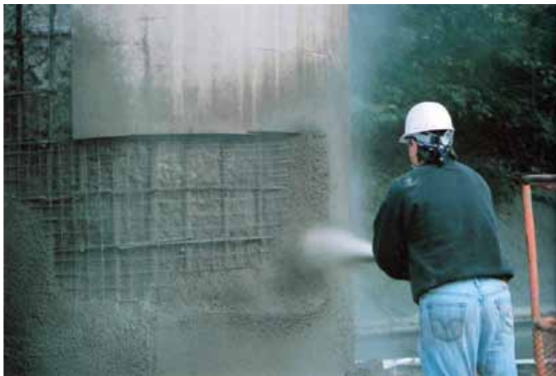
Nozzleman gunning dry-process shotcrete—filling the edges of the repair area first—and working toward the middle to avoid trapping rebound in the corners
