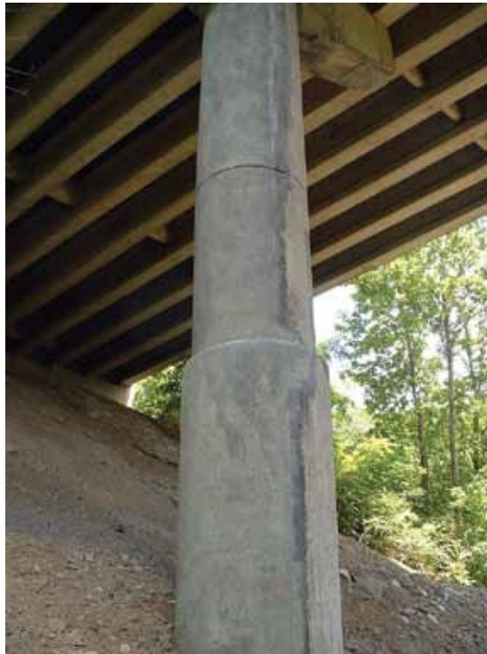
Shotcrete easily conforms to the circumference of this round bridge pier and works well with irregular shapes and configurations
