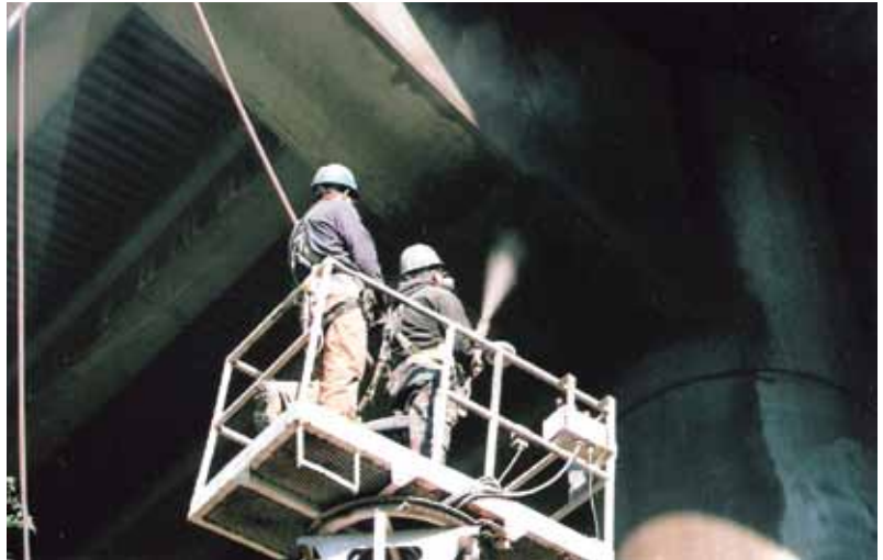
Overhead dry-process shotcrete being placed on the underside of a pier hammerhead in Pittsburgh, PA
