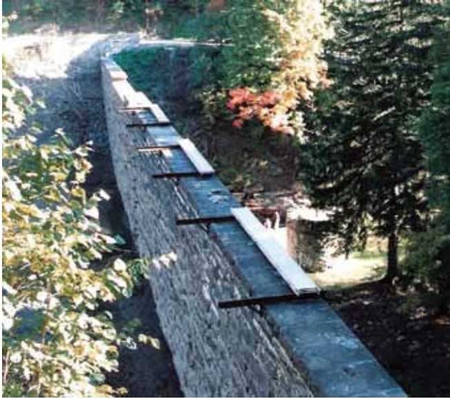
Outriggers in place across the top of a dam with stages positioned to be rigged
