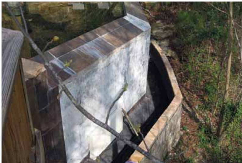
Efflorescence vanishing edge (another view)
