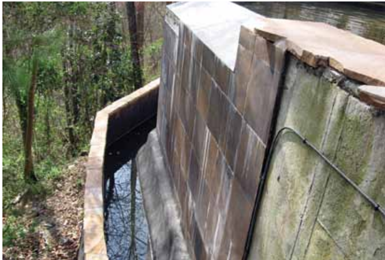
Efflorescence vanishing edge
