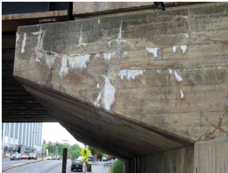
Bridge abutment deterioration
