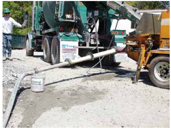
Fig. 8: Pump with multiple reducers
