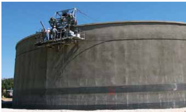
Fig. 2: Wrapping prestressing wire on circular prestressed tank Photo courtesy of Preload Company
