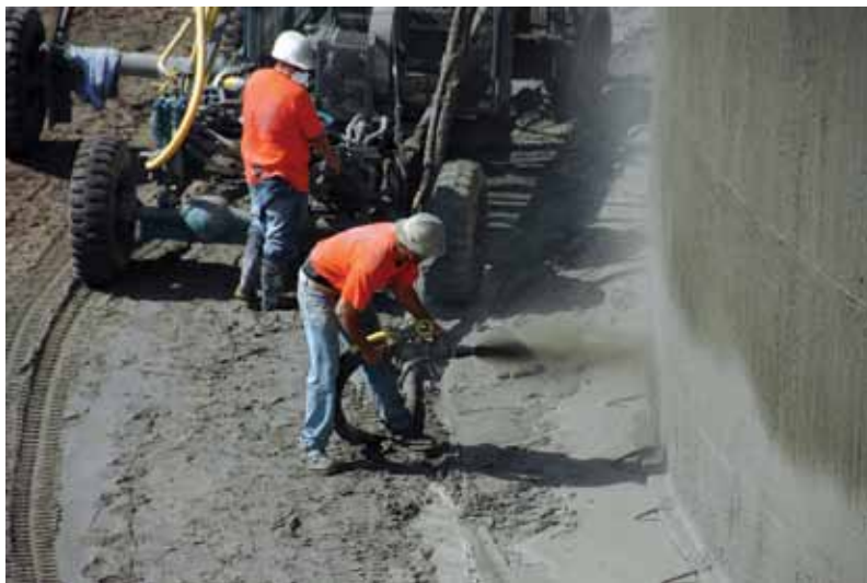
Fig. 4: Shooting core wall at the base of the tank Photo courtesy of Crom Corporation
