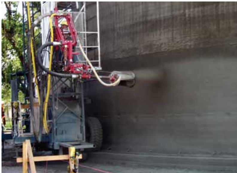
Fig. 5: Remotely controlled shotcrete nozzling of tank wall Photo courtesy of Crom Corporation
