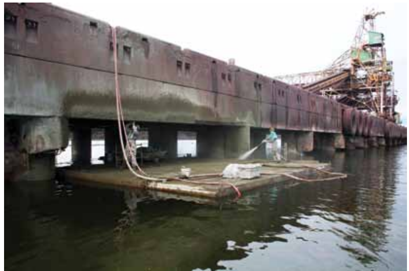
Barge platform supporting both a finisher and a nozzleman, working in tandem to complete the repair patch before moving to another area
