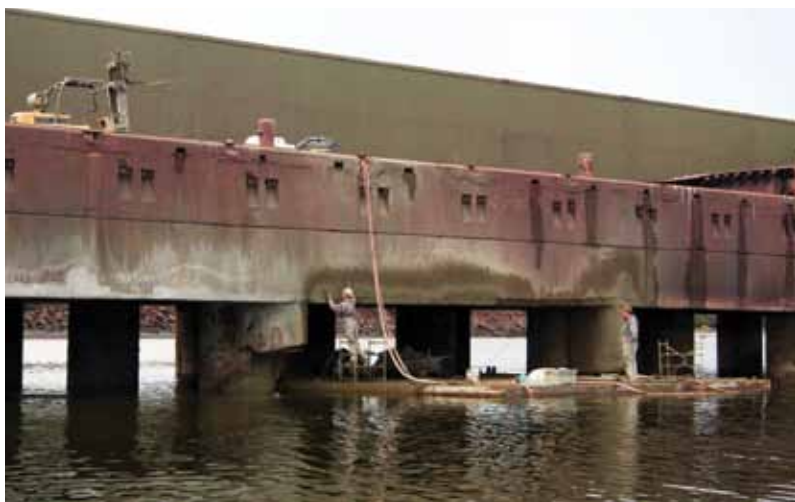
A finisher is completing the repair with a trowel while a fork-lift and some of the shotcrete equipment remain on top of the wharf, allowing efficient resupplying while creating more space
