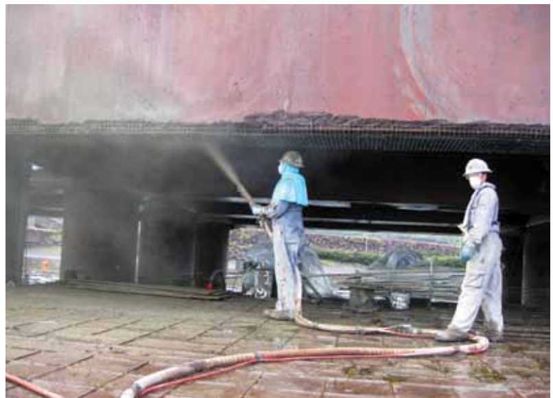
Nozzleman applying the initial coat of shotcrete to a repair 3 to 6 in. (75 to 150 mm) deep using the dry-mix process during high tide
