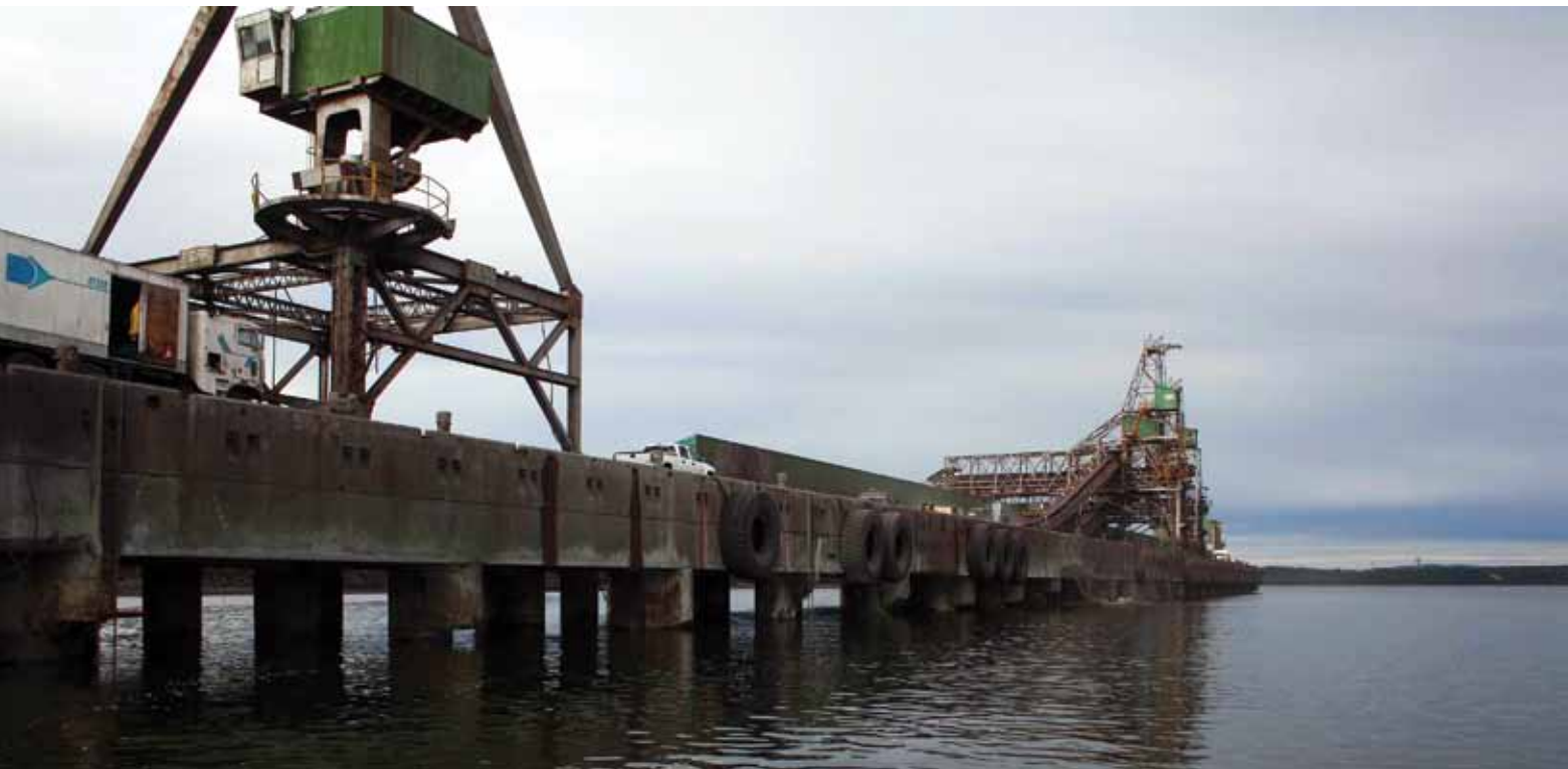
Wabush Wharf extending into a cove near Sept-Îles. Loading cranes and supply trucks are also visible on top of the 60-year-old concrete structure
