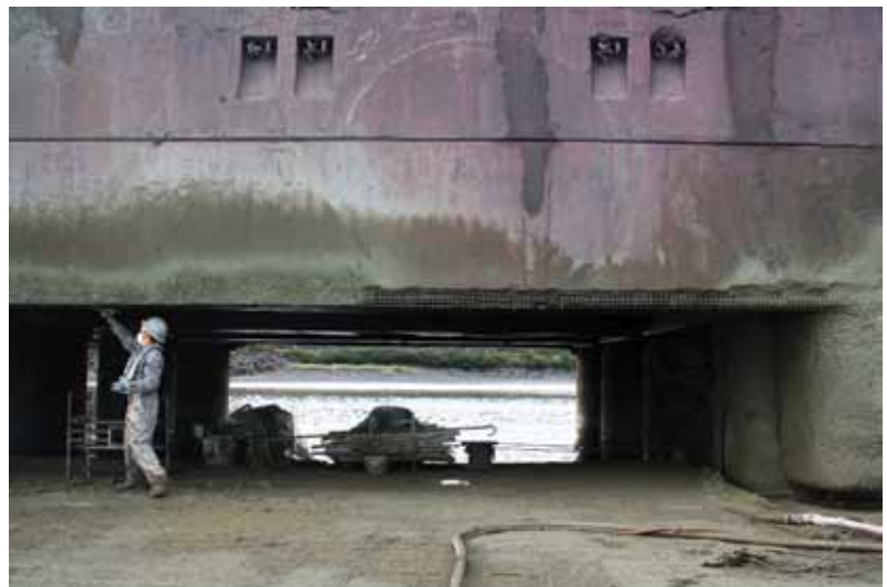
Concrete finisher creating an edge on the repair patch during high tide. The securely fastened metallic trellis can be seen in the uncompleted section
