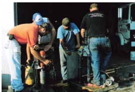
The core drilling of the shotcrete panels to see the encapsulation of the reinforcing bar
