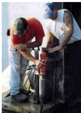
The core drilling of a shotcrete panel to see the encapsulation of the reinforcing bars
