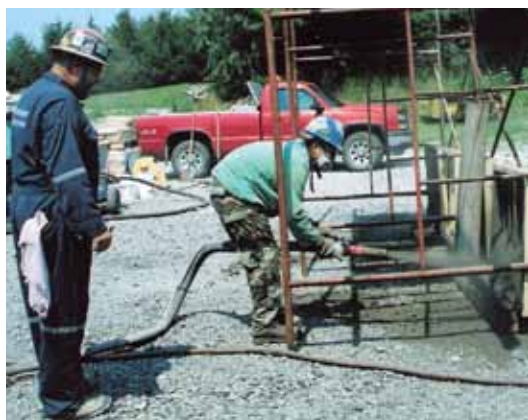
The gunning of a vertical panel with Examiner Ray Schallom looking on
