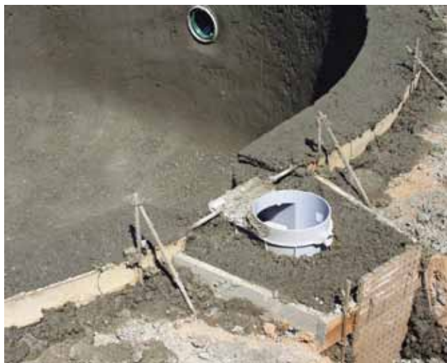
Typical bender board form work around a swimming pool that sets the shape, elevation, and dimensions
