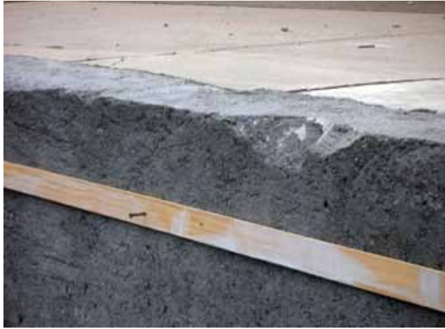
Batter board attached to the pool shell with concrete nails. Note the minor damage to the top of the pool wall
