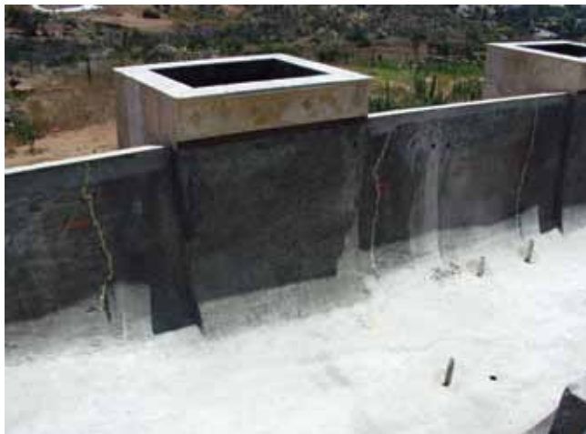
Vanishing edge weir wall where shrinkage cracks reflected through water line tile. Repair was by epoxy injection
