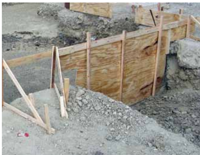
After shotcrete, backfilling of the pool wall will be necessary before work on the pool can continue
